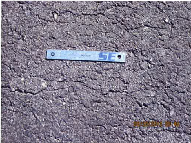
R-1, Surface detail with cracking
