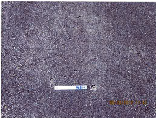
T-4, Surface detail with raveling
