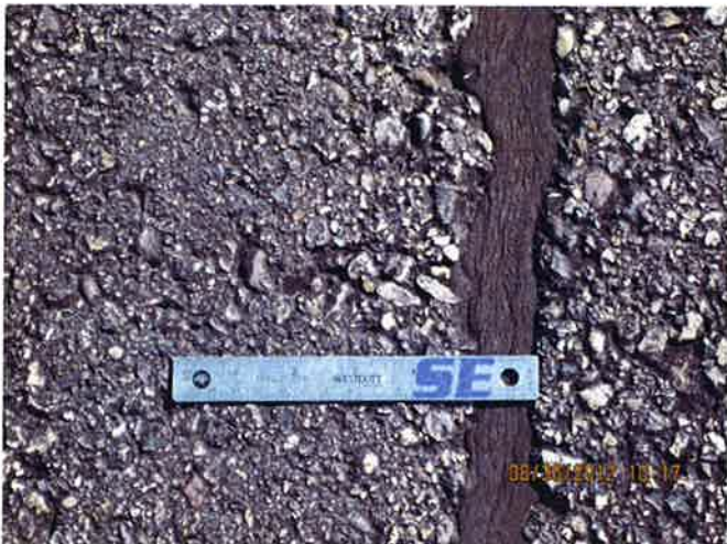
R-2, Surface detail with crack
