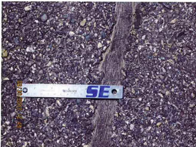
T-2, Surface detail with crack
