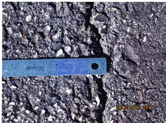
R-1, Surface detail with crack
