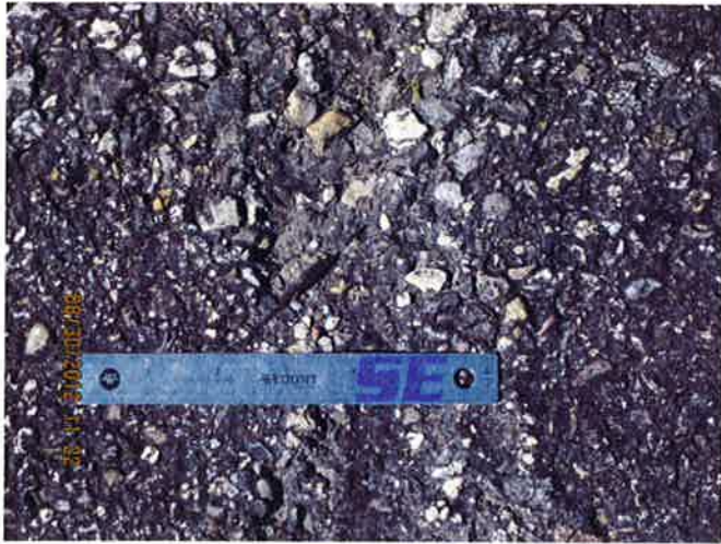
T-3, Surface detail with raveling
