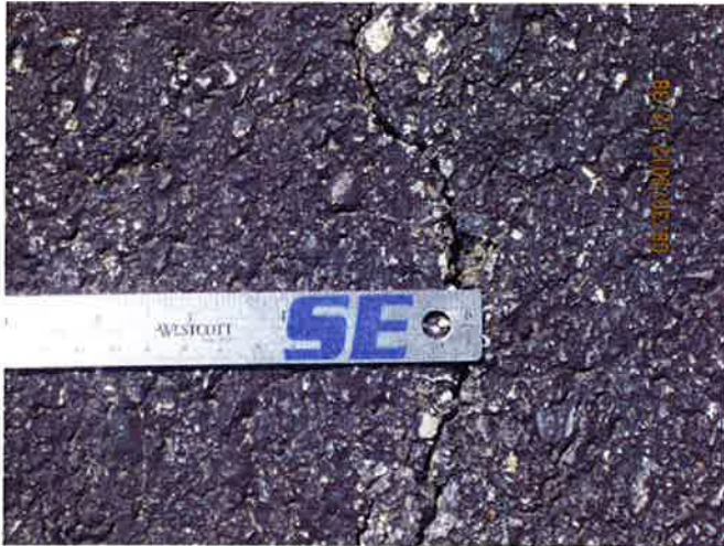
T-1, Surface detail with crack
