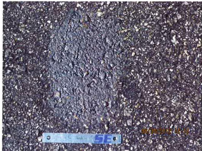
A-2, Surface detail with oil spillage
