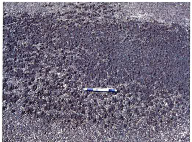
R-4, Surface detail with bleeding
