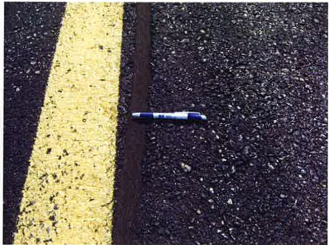
T-3, Surface detail with crack
