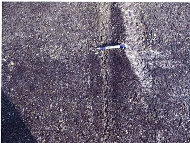
A-11, Surface detail with crack
