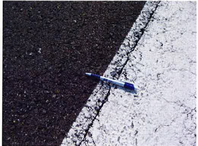
R-21, Surface detail with crack
