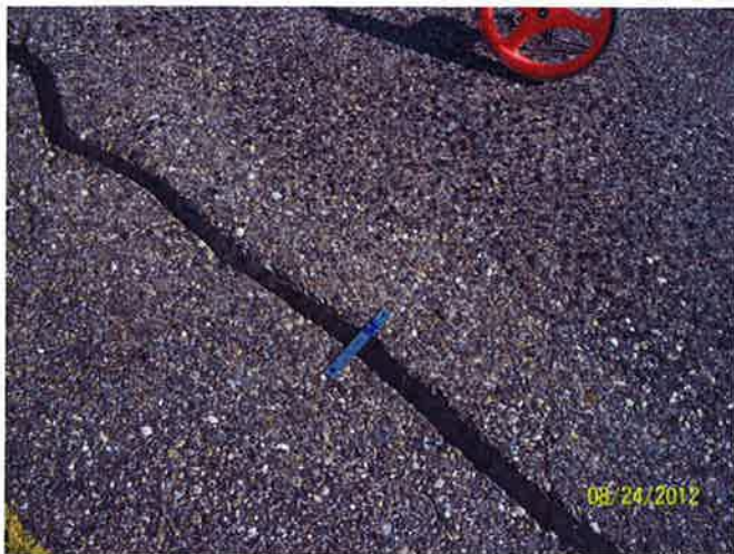
T-2, Surface detail with cracking and bleeding
