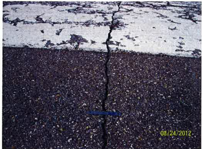
R-1, Surface detail with cracking
