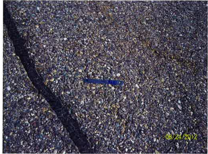
A-1, Surface detail with raveling and cracking
