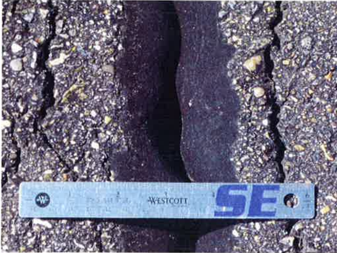
T-3, Surface detail with crack
