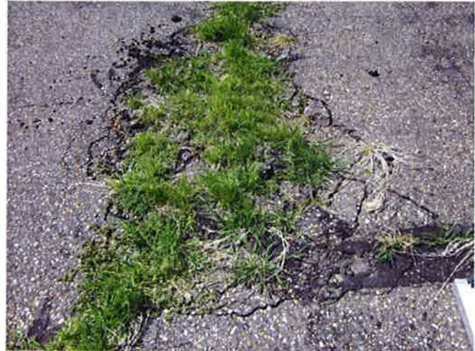
T-3, Surface detail with depression and cracking
