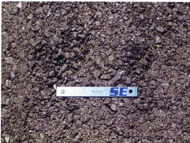
T-2 , Surface detail with raveling
