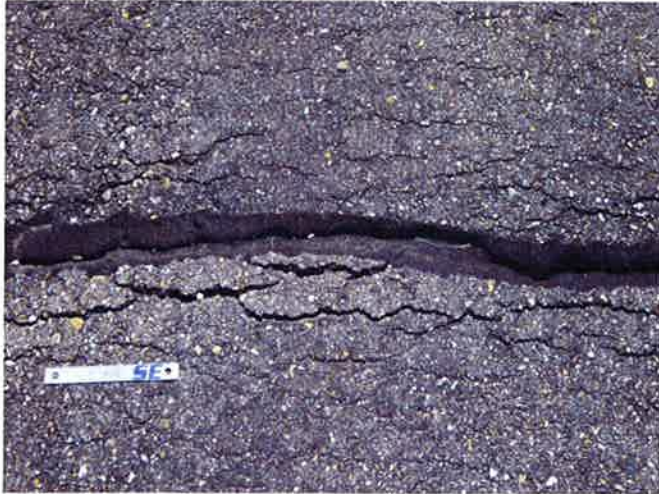
T-1 , Surface detail with cracking
