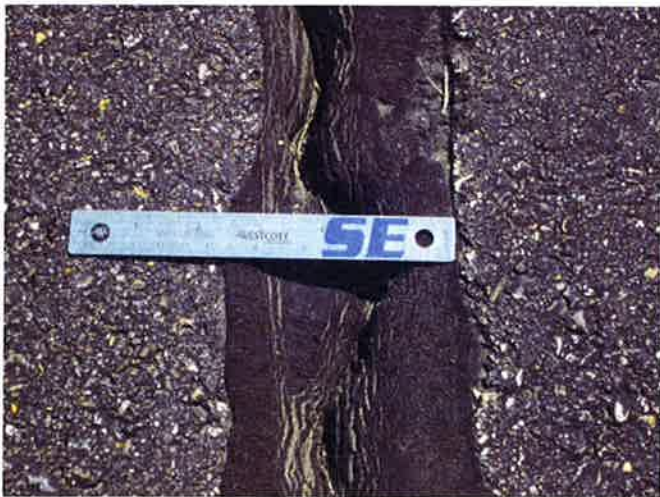
R-1, Surface detail with crack
