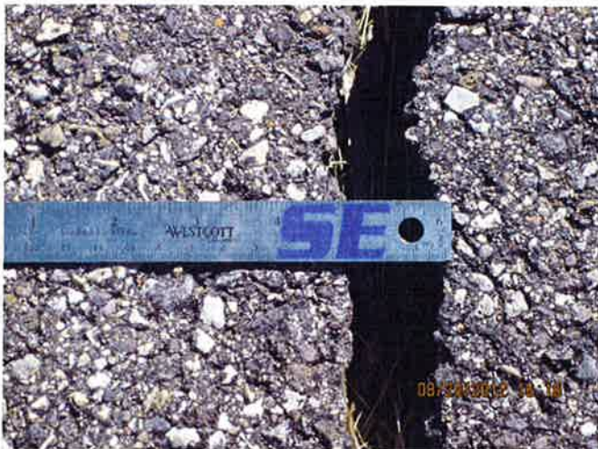
R-1, Surface detail with crack
