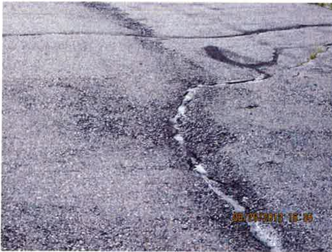
T-1, Overview with crack and raveling
