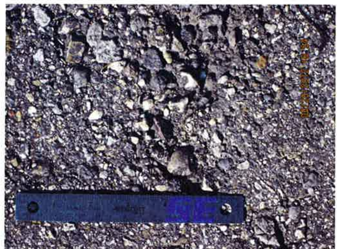
R-1, Surface detail with raveling
