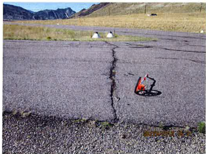
T-1, Overview with crack
