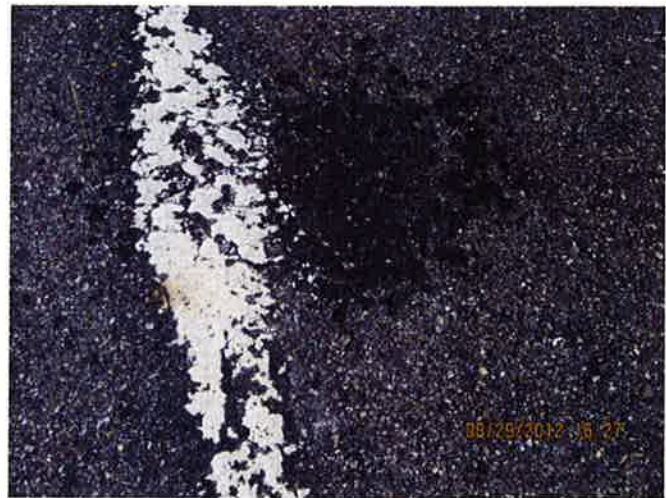
R-1, Surface detail with bleeding
