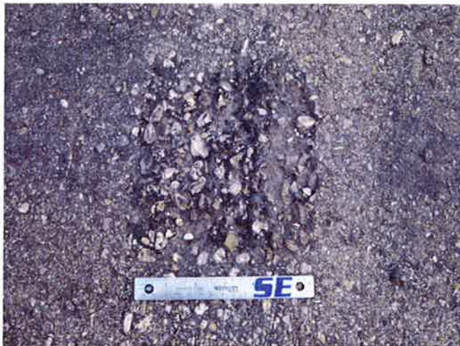
A-11, Surface detail with raveling
