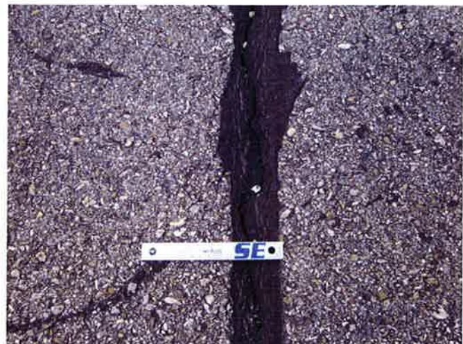
T-11, Surface detail with crack
