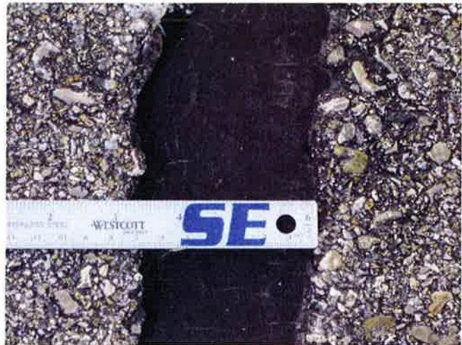
A-11, Surface detail with crack
