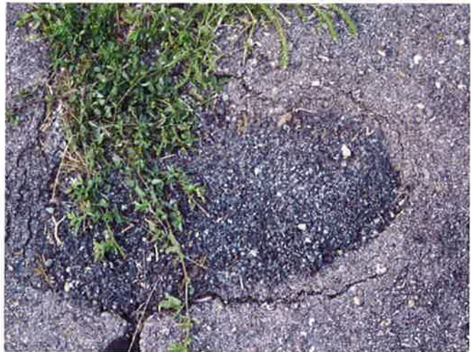
R-11, Surface detail with patch
