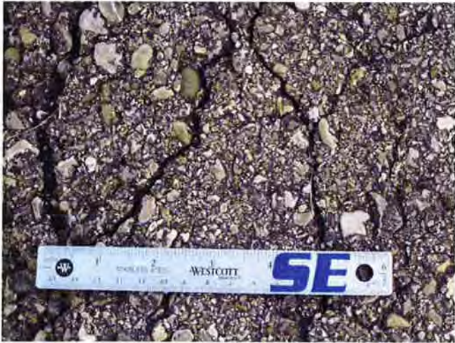
T-11, Surface detail with cracking
