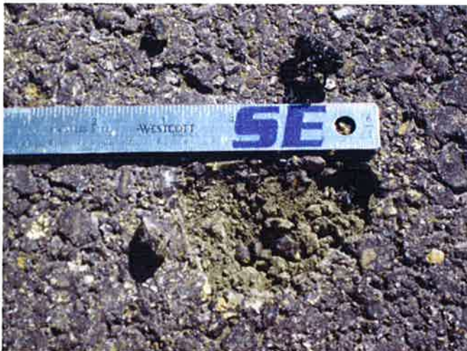
T-1, Surface detail with raveling
