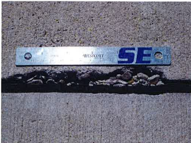
A-3, Surface detail with spalling
