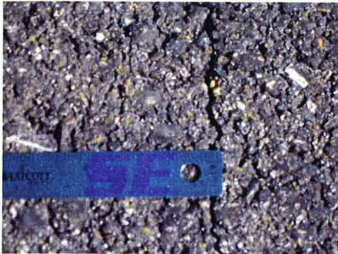
R-1, Surface detail with crack
