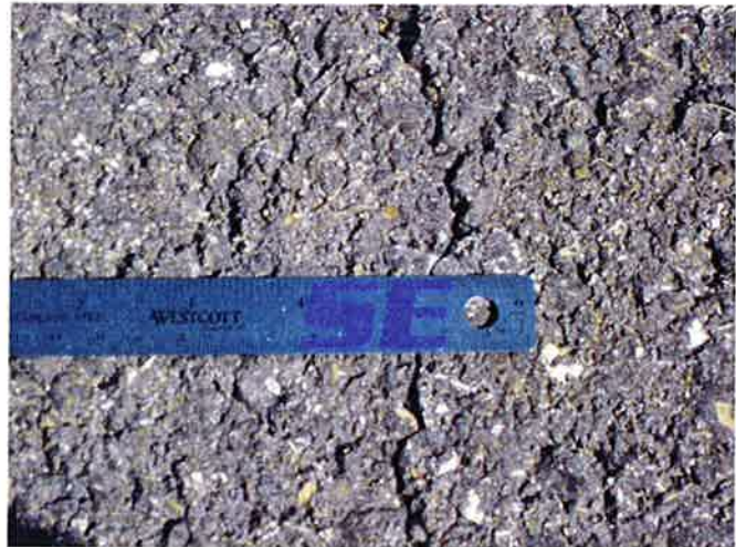
A-1, Surface detail with crack
