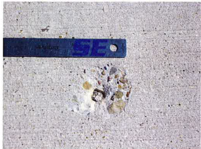
A-3, Surface detail with scaling
