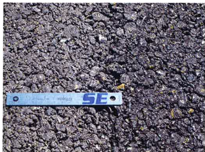
R-1, Surface detail with raveling
