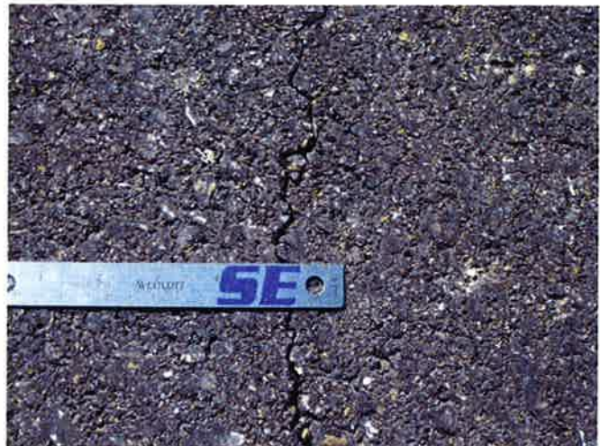
T-1, Surface detail with crack
