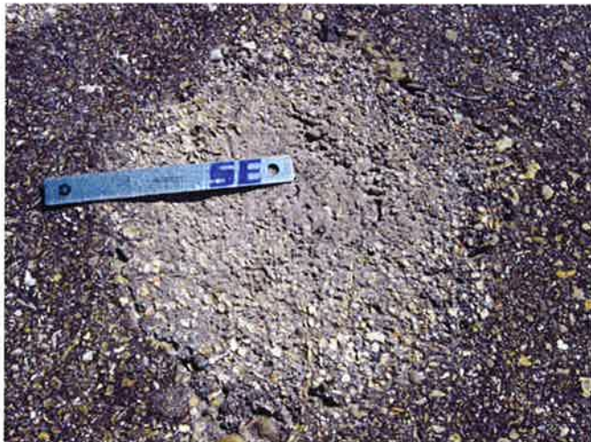
T-2, Surface detail with patch
