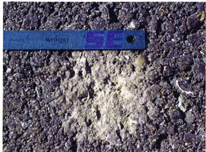
T-2, Surface detail with raveling
