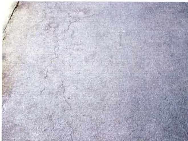
A-1, Surface detail with cracking
