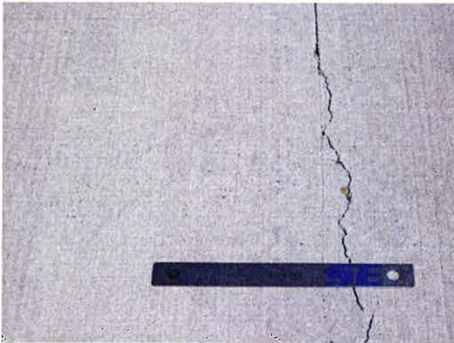
A-3, Surface detail with crack
