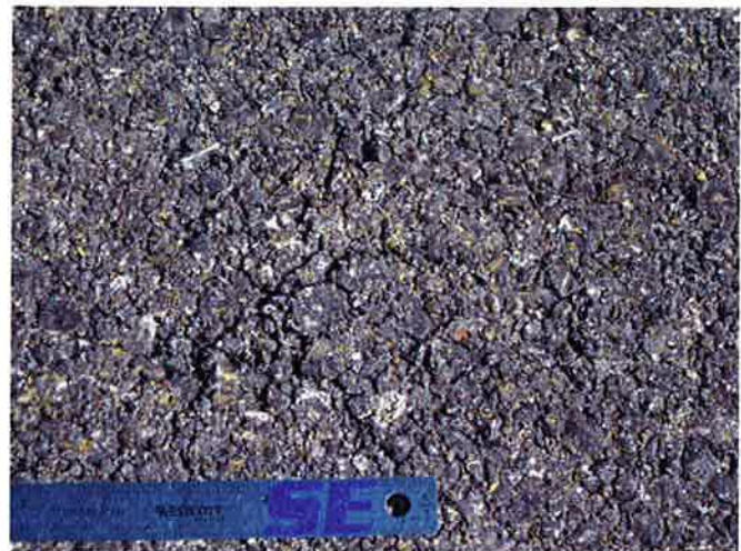
R-1, Surface detail with cracking
