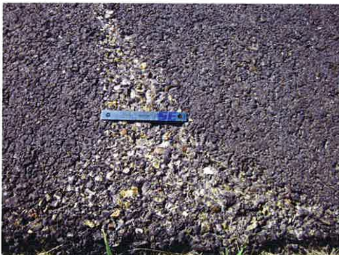
R-1, Surface detail with raveling 2
