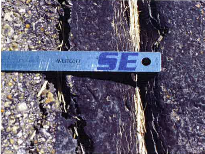
T-2, Surface detail with crack
