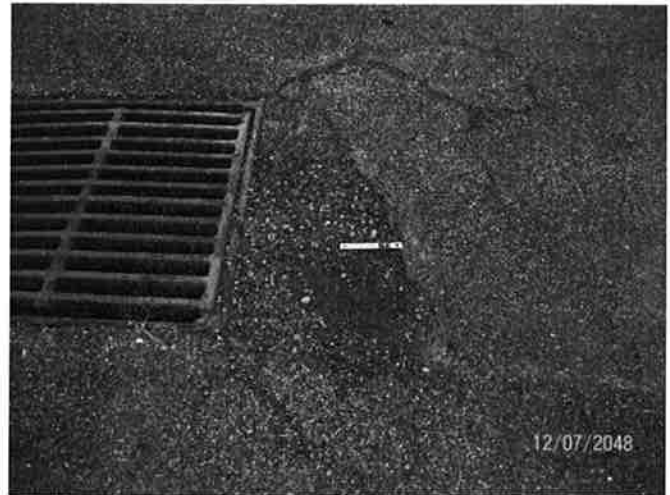
A-2, Surface detail with raveling
