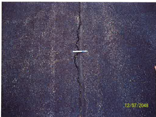
A-3A, Surface detail with cracking
