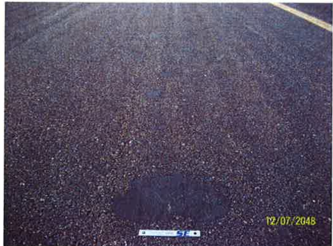
T-3B, Surface detail with bleeding
