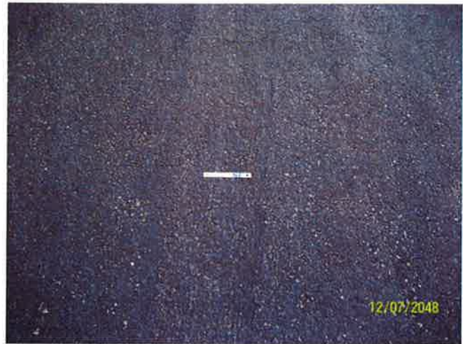
T-3, Surface detail with raveling from paint obliteration
