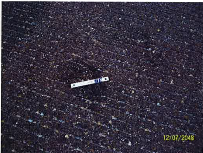
R-12, Surface detail raveling from lock wheel turn
