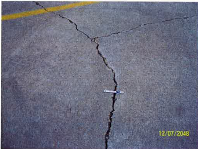
A-5, Surface detail shattered slabs
