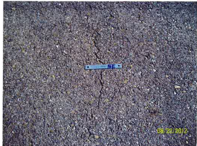
T-1, Surface detail with cracking
