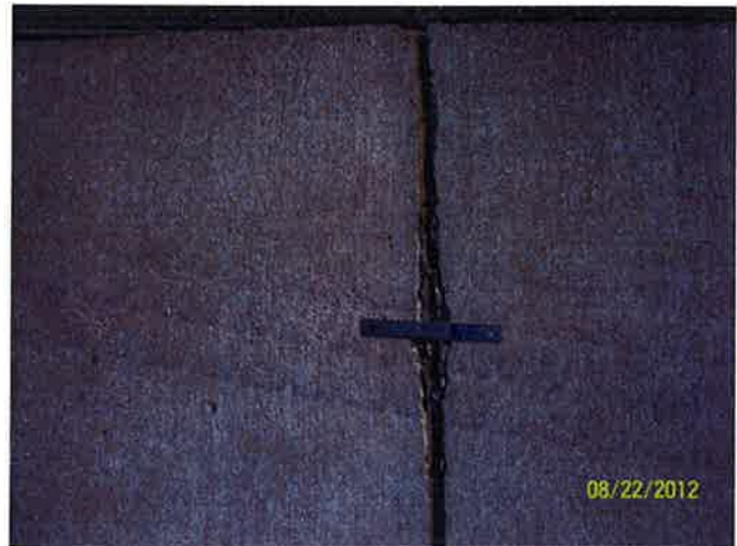
A-3, Surface detail with joint spalling
