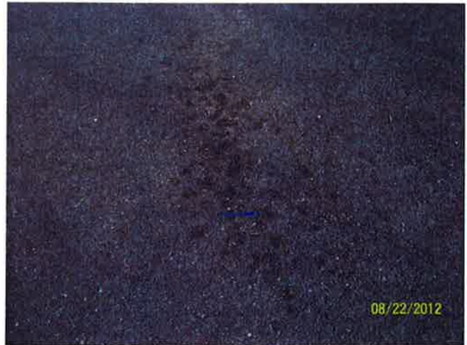
A-1, Surface detail oil spillage
