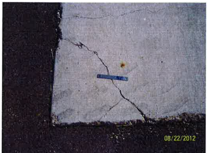
A-2, Surface detail with cracking and corner break
