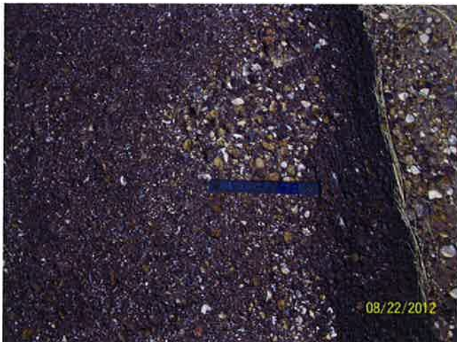
T-3, Surface detail raveling from snow plow damage
