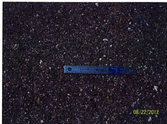
R-1, Surface detail with cracking
