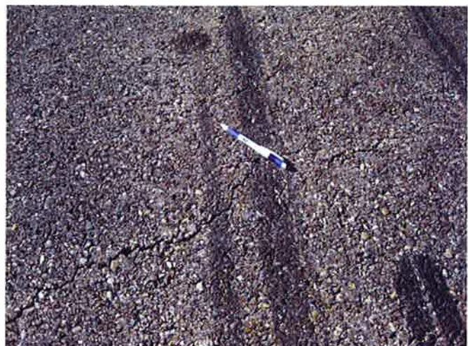
R-11, Surface detail with cracks
