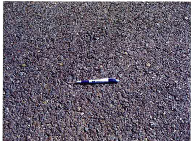
A-11, Surface detail with weathering
