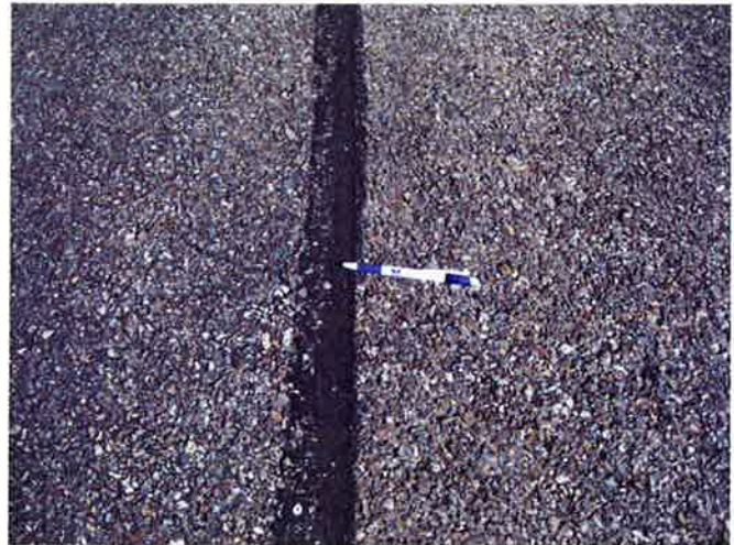
T-4, Surface detail with cracks
