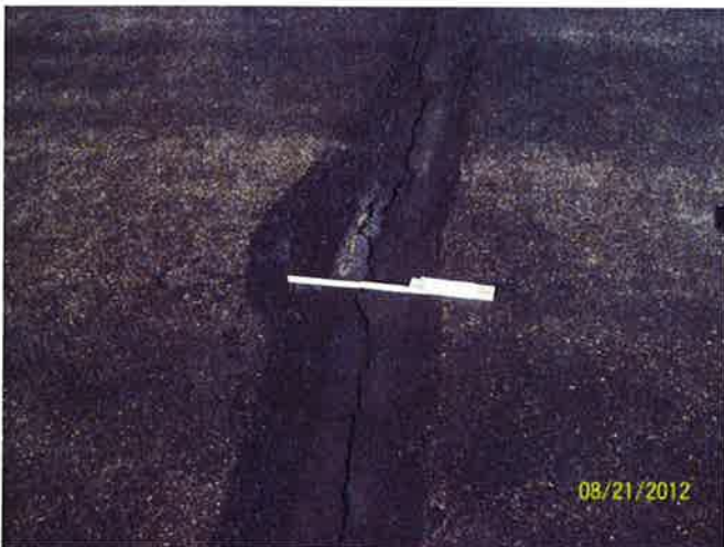
T-11, Surface detail with cracked crack repair
