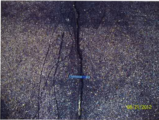
T-13 , Surface detail with cracking
