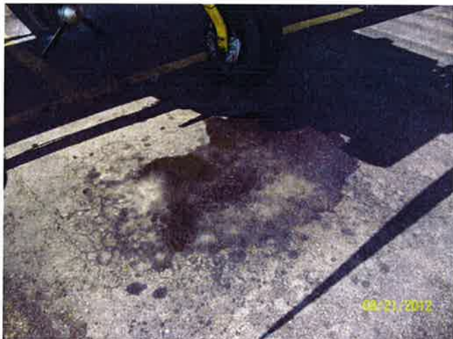
A-12, Oil spillage
