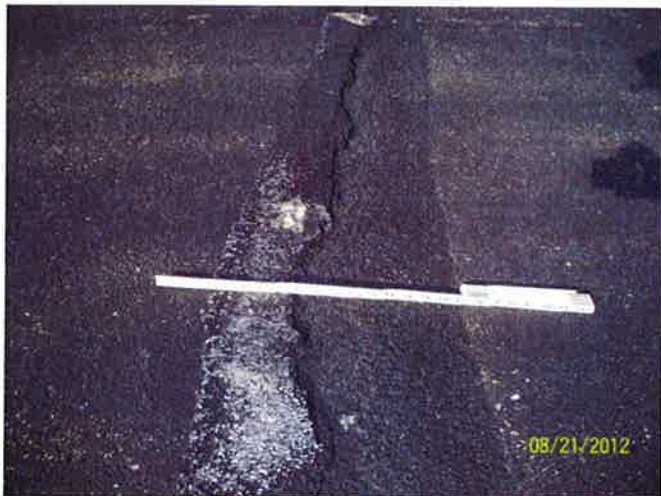
R-11, Surface detail with cracked crack repair
