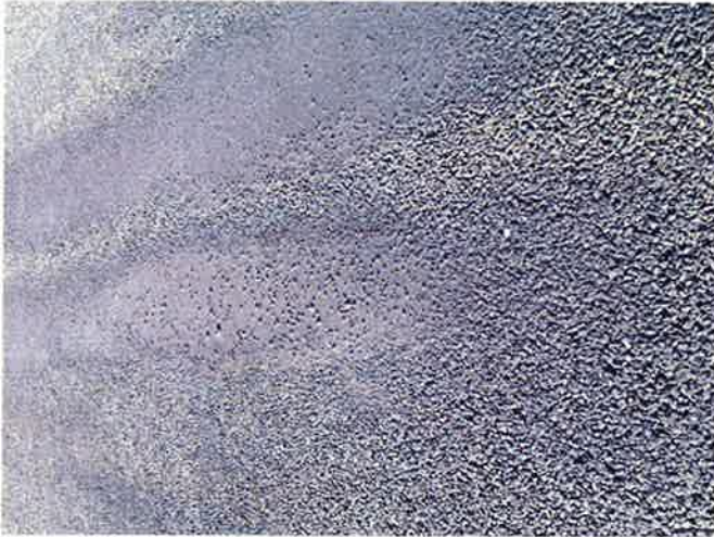
R-1 , Surface detail with bleeding
