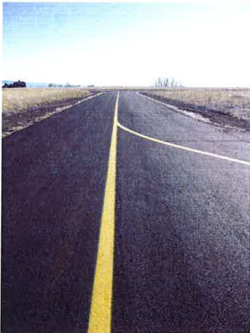
T-3 , Overview with crack
