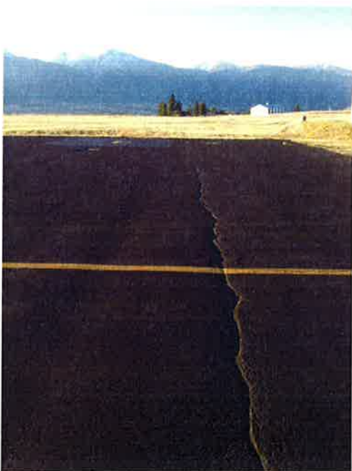
A-2, Overview with crack
