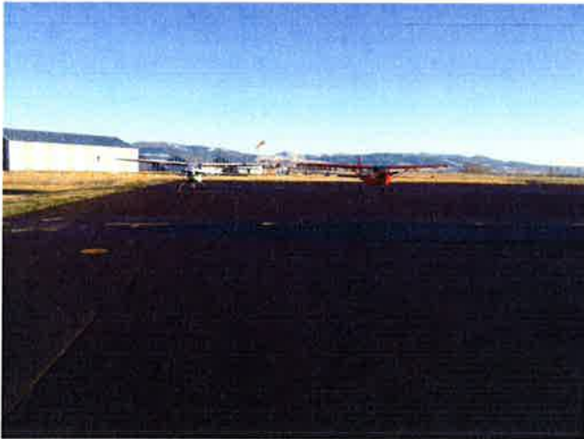
A-1, Overview crack
