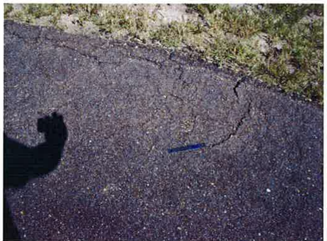
T-11, Surface detail alligator cracking
