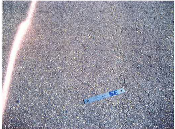
R-11, Surface detail alligator cracking
