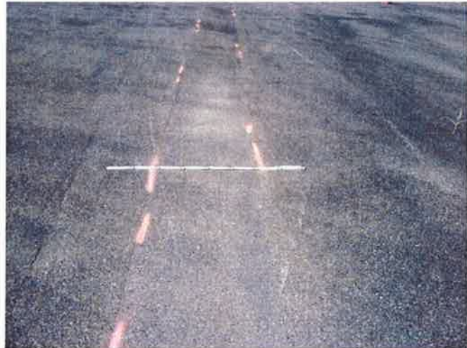
A-11, Surface detail depression
