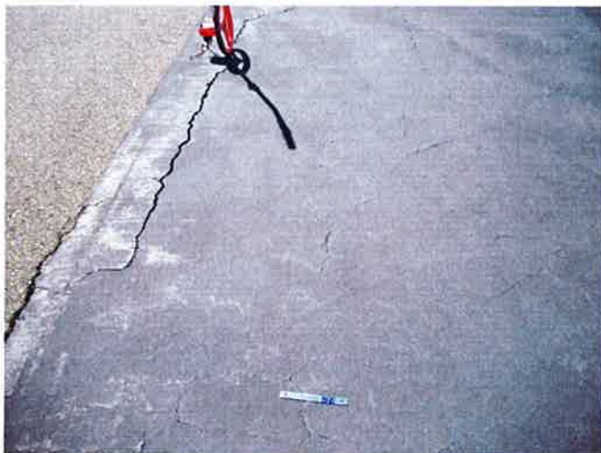
A-11, Surface detail raveling coal tar and cracking
