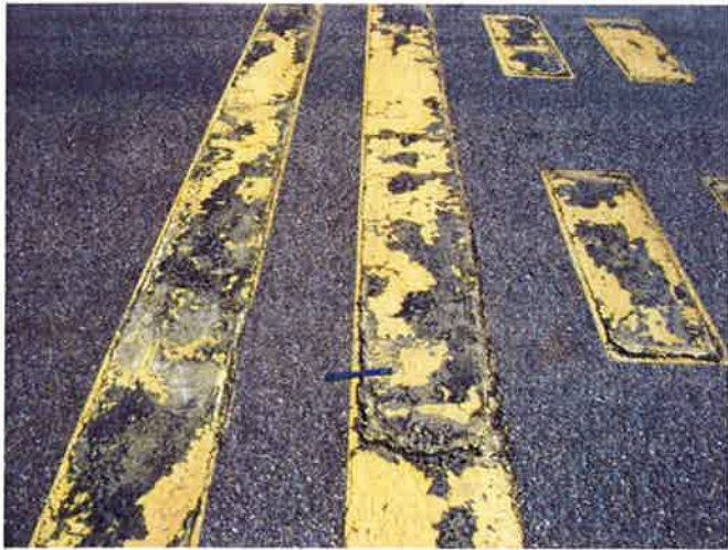
T-11, Surface detail cracking at painted markings
