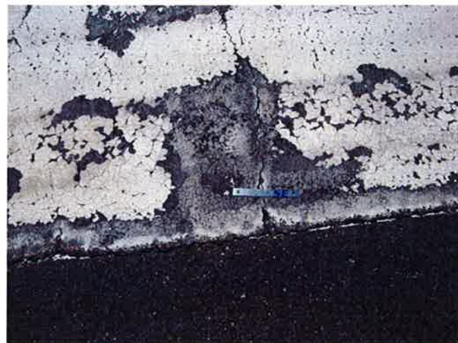
R-11, Cracking around numbers
