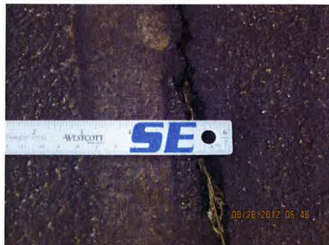
R-1, Surface detail with crack
