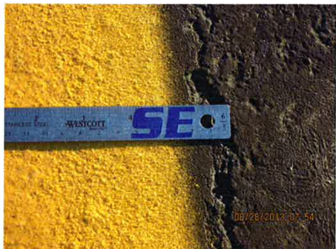
T-1, Surface detail with crack
