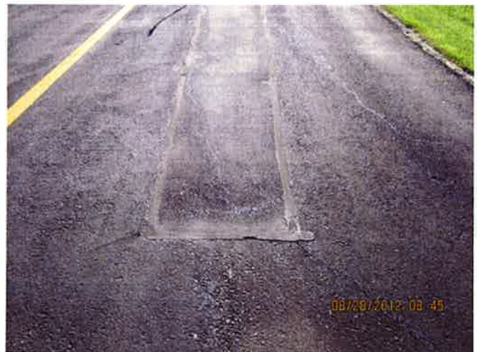
T-2, Surface detail with patch
