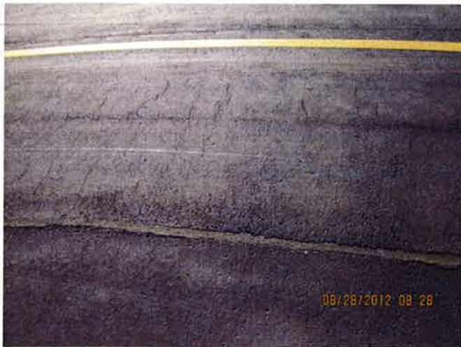
T-1, Surface detail with cracking
