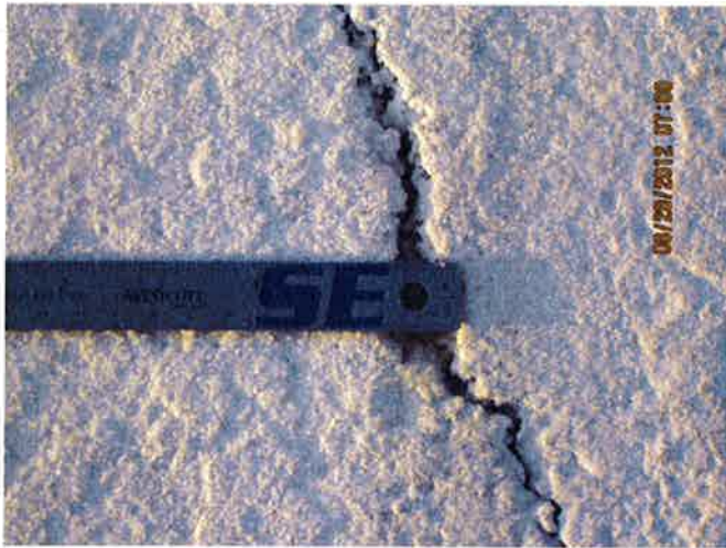
R-1, Surface detail with crack 2
