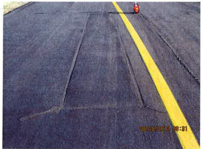
T-1, Surface detail with patch
