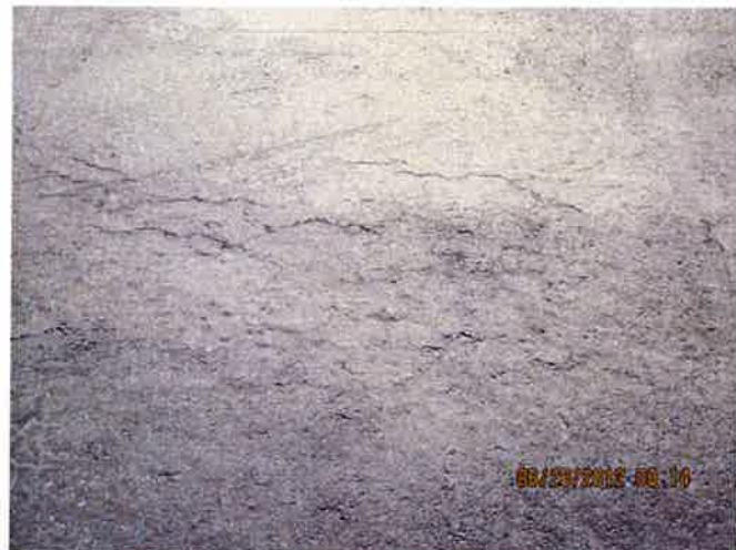
A-1, Surface detail with cracking 2
