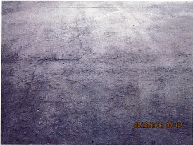
A-1, Surface detail with cracking
