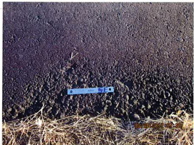
R-1, Surface detail with raveling
