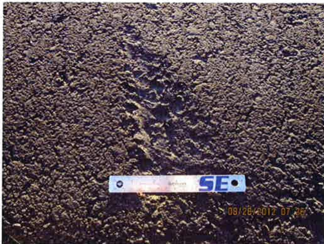
R-1, Surface detail with raveling 2
