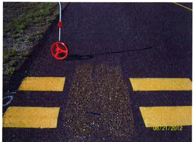
T-1, Surface detail raveling from paint obliteration
