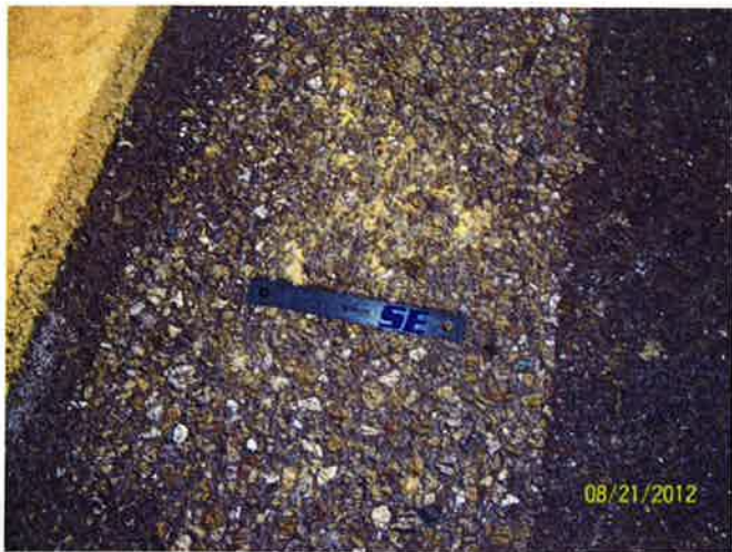
T-3, Surface detail raveling from paint obliteration
