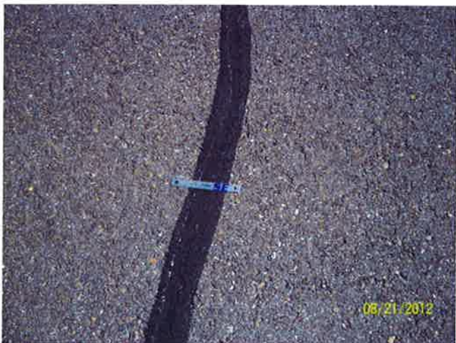
T-4, Surface detail with cracking
