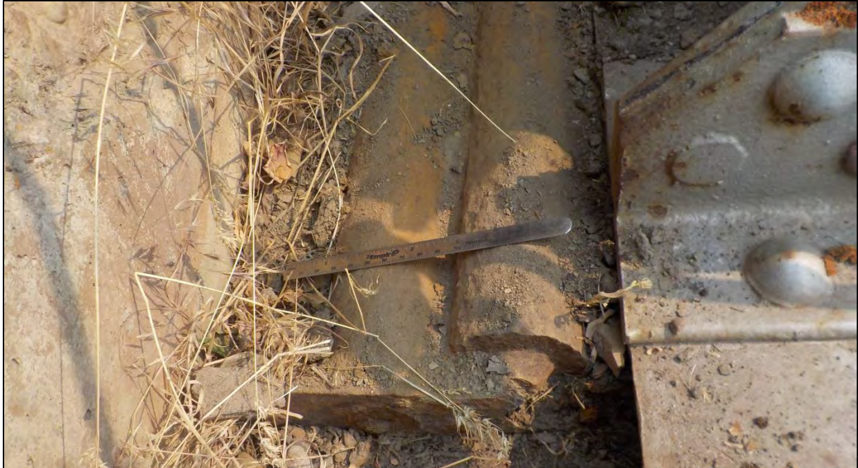
Photo 62: Abutment 1, North Truss roller bearing with two of the rollers severed and displaced from underneath the roller keepers
