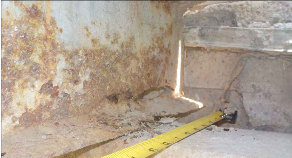
Photo 52: Span 2, Bent 3, Stringer 4: the stringer web had heavy corrosion and section loss with a 5 in. long by 1 in. high through hole near the stringer end. The bottom flange was knife edges in this area
