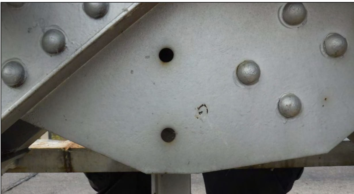
Photo 75: Span 2, North Truss, Gusset Plate U1': the exterior gusset plate had two misdrilled 3/4 in. diameter holes
