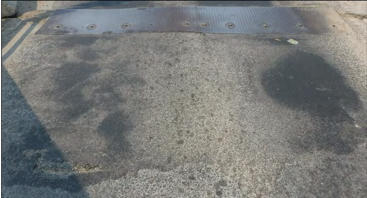
Photo 24: End 6 ft. at the West Transition had cold patch with minor wear and hairline map cracking
