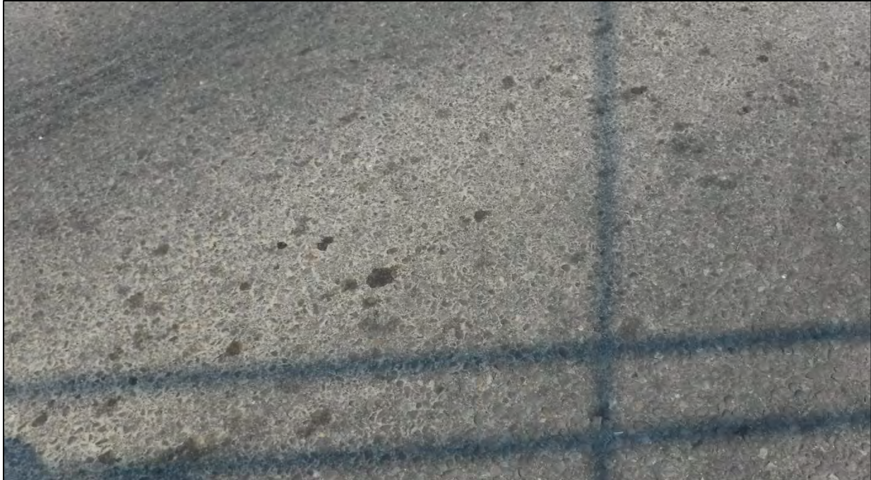
Photo 22: Typical minor wear on Span 1 bituminous overlay
