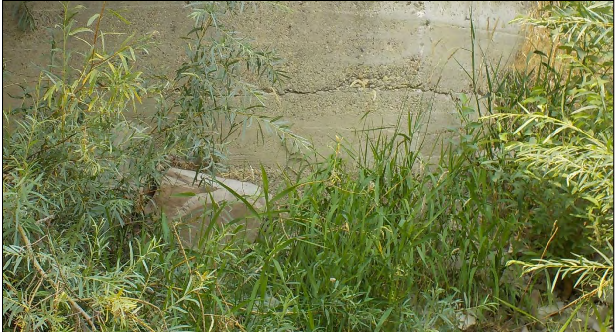
Photo 58: Bent 3 had a 5 ft. long horizontal crack up to 1/16 in. wide was located near the bottom, northeast corner
