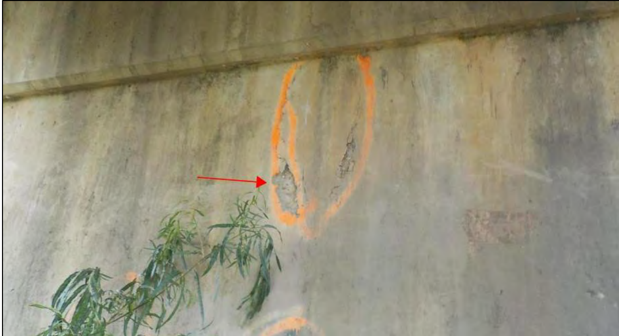
Photo 56: Bent 2 with areas of spalling on the edge of a delamination with 1 in. of penetration and no exposed reinforcing steel
