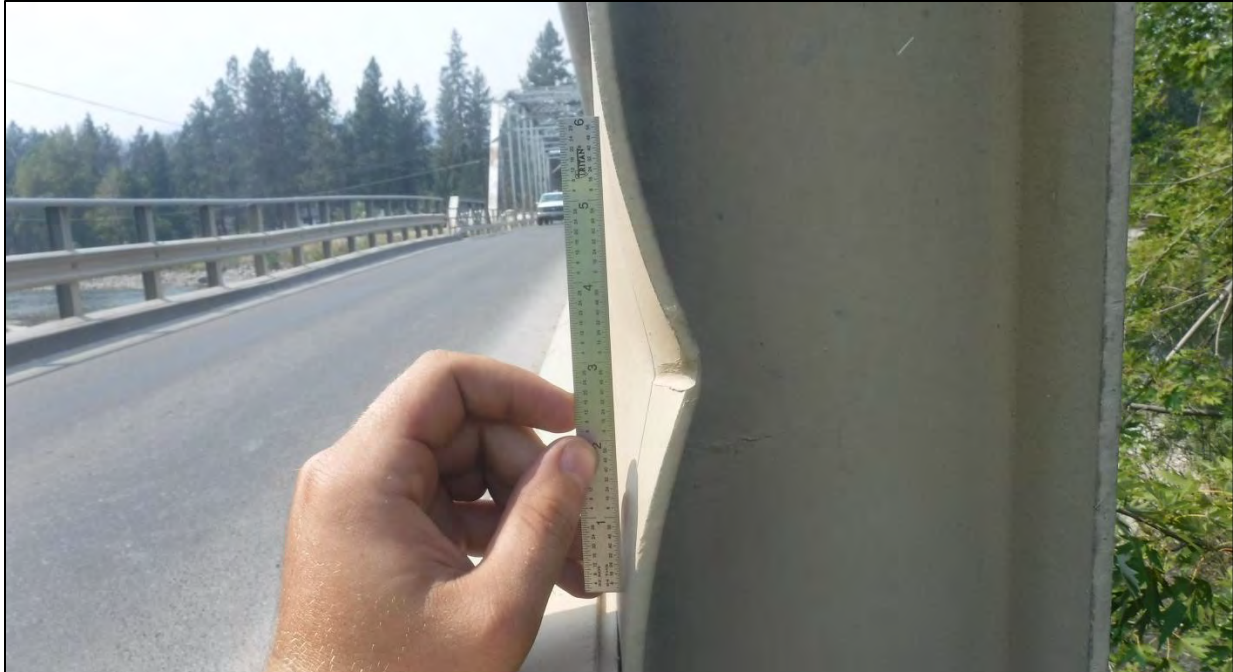
Photo 36: Three vertical members had impact damage that bent the interior flange 3/4 in. over a 6 in. length on the North Rail near the East Approach
