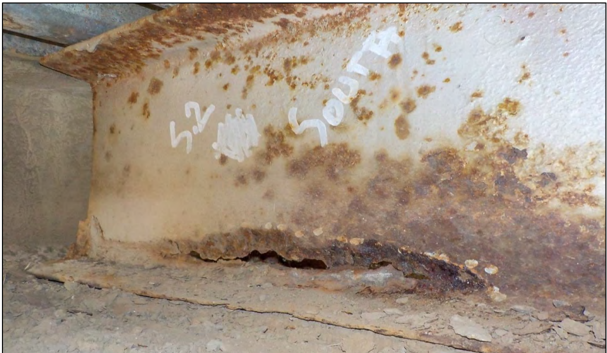
Photo 45: Span 1, Abutment 1, Stringer 2: the stringer web had heavy corrosion and section loss over a 17 in. long by 2 in. high area with a 1 in. diameter hole center 10 in. from the stringer end
