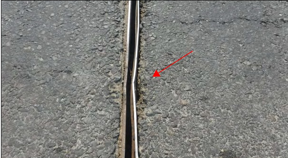
Photo 42: Joint 3 over Bent 3 with separation from the Span 2 deck over a 4 ft. length
