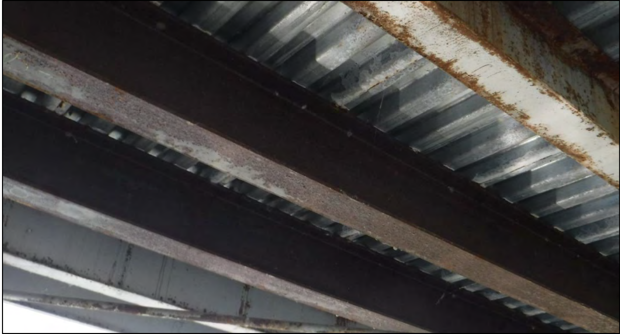
Photo 44: Typical unpainted stringers with minor to moderate corrosion and negligible section loss
