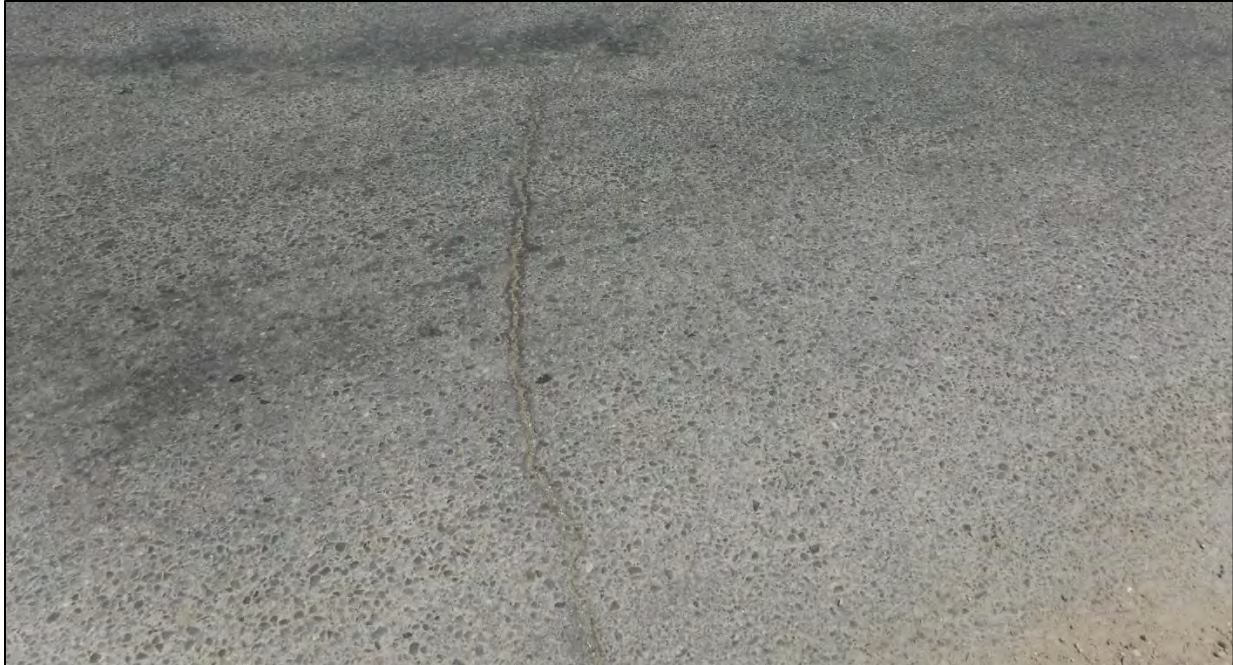
Photo 20: 1/4 in. wide transverse crack located 18 ft. from the West Transition
