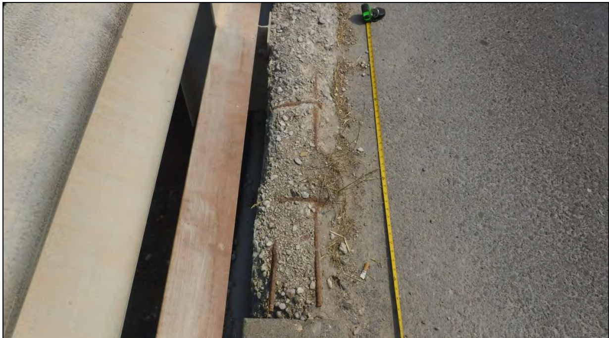
Photo 31: The North Curb had section loss up to 5 in. with exposed longitudinal and stirrup reinforcing steel for 4 ft. over Bent 4
