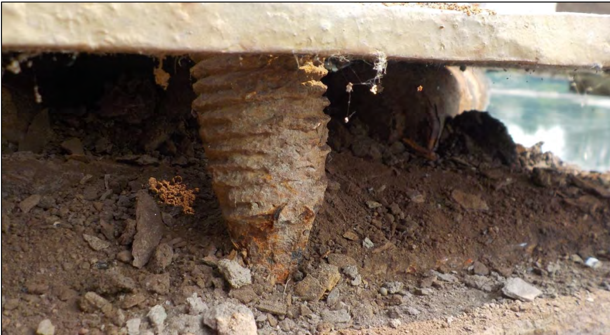
Photo 61: Abutment 1, North Truss roller bearing with heavy corrosion and section loss to the anchor rods
