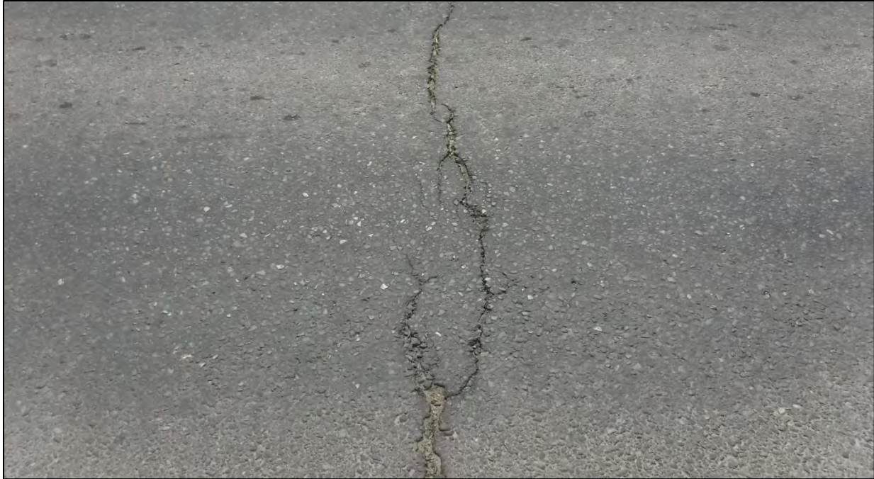
Photo 26: Transverse crack up to 1/2 in. wide over Bent 4
