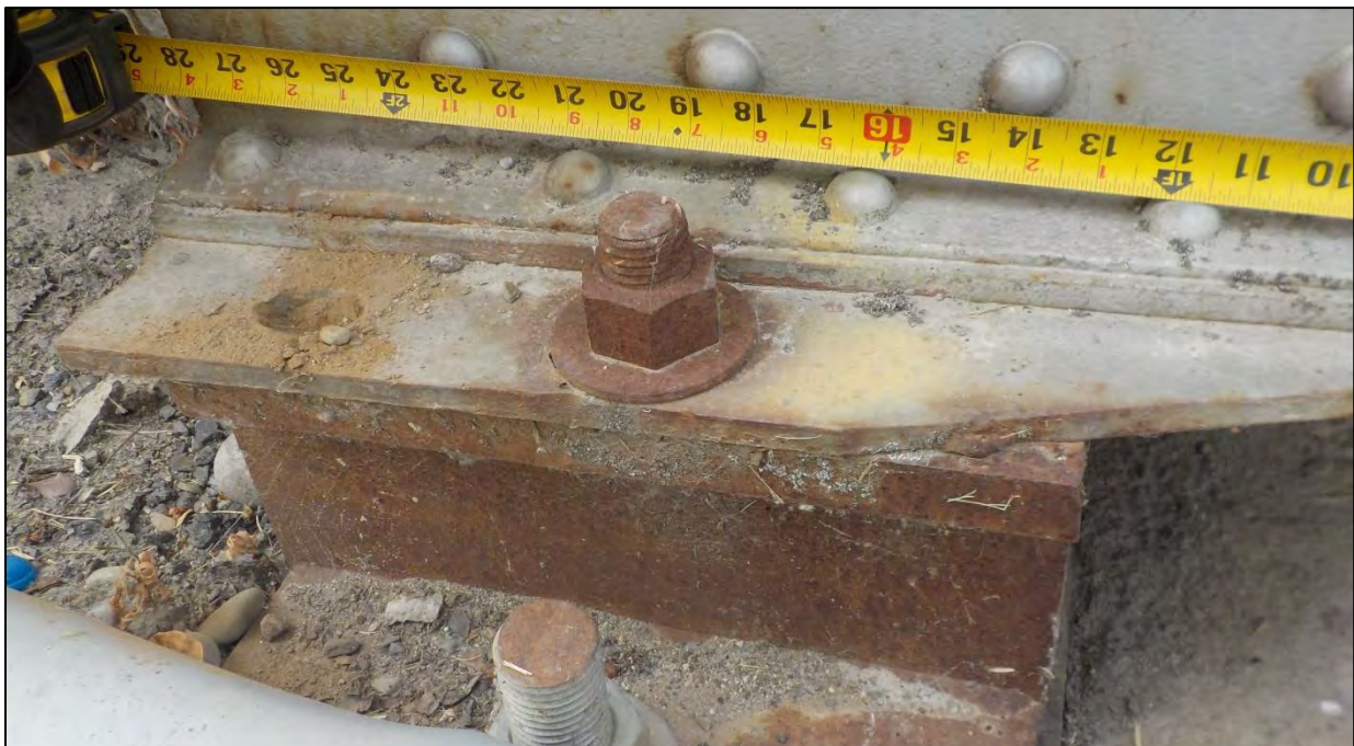
Photo 69: Bent 3, North Truss, Span 2 slider bearing
