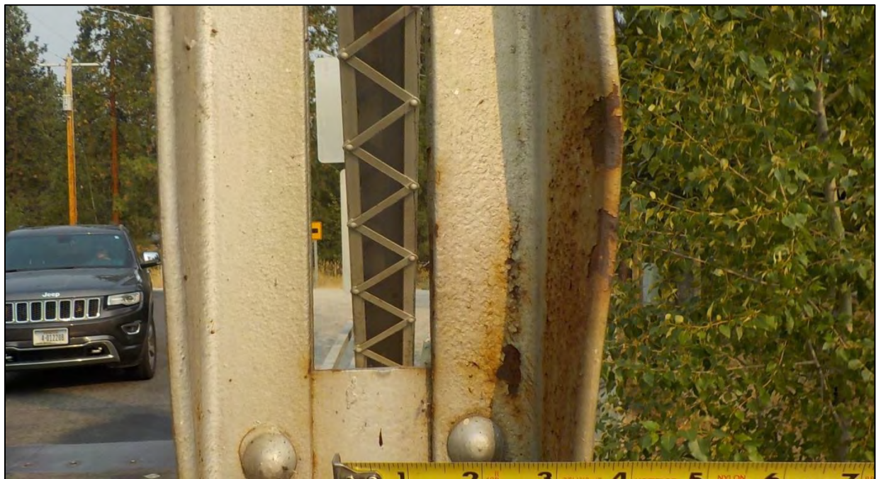
Photo 71: Span 1, North Truss, Vertical U1-L1: the exterior flange of the vertical was bent 1 in. to the north due to impact damage approximately 5 ft. above the bridge deck
