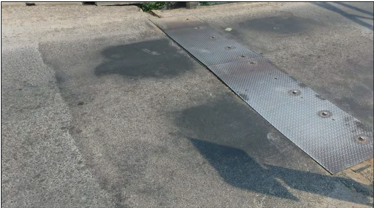
Photo 19: West Approach within 5 ft. of bridge deck had section of cold patch in good condition
