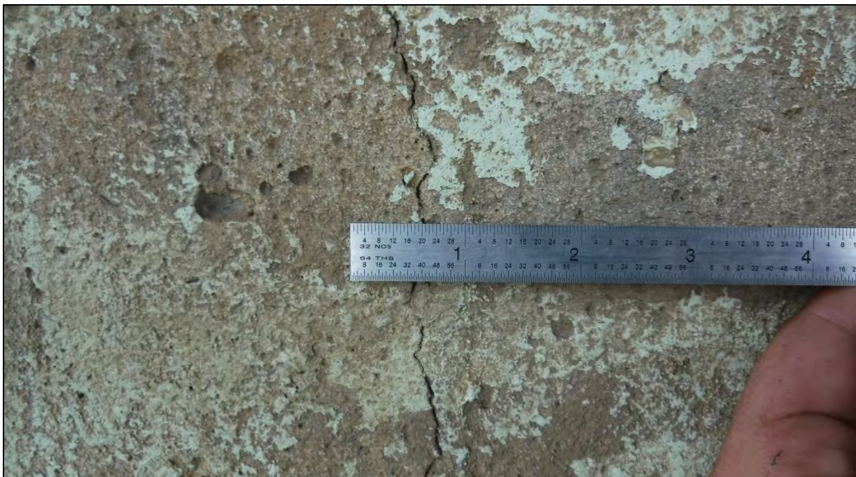
Photo 55: Abutment 1 had one full height, vertical up to 1/8 in. wide in the middle of the abutment
