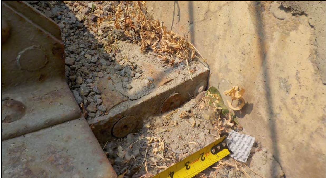
Photo 64: Abutment 1, South Truss roller bearing with the rollers and roller keeper protruding out from underneath the bearing and resting against the abutment backwall
