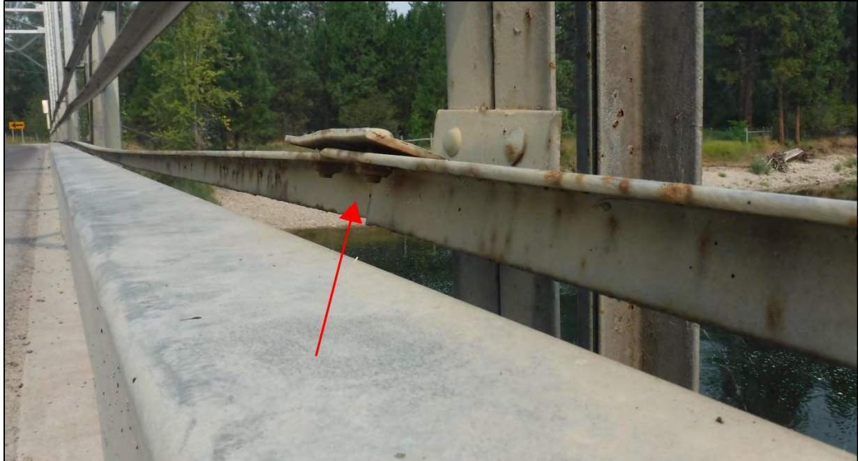
Photo 34: North Rail, Panel Point 1': The bottom angle was bent 3/4 in. upwards
