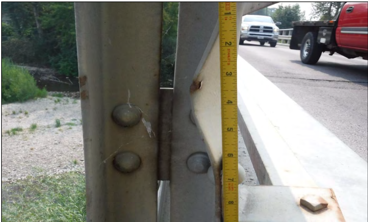
Photo 73: Span 2, North Truss, Vertical L2'-U2': the interior flange of the vertical was bent 1 in. over a 6 in. length due to impact damage
