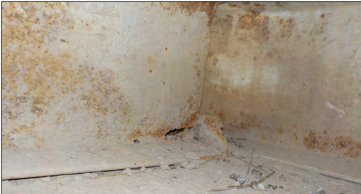
Photo 47: Span 1, Abutment 1, Stringer 7: the stringer web had heavy corrosion and section loss over a 14 in. long by 2 in. high area with a 2 in. long by 1/2 in. high hole center 2 in. from the stringer end
