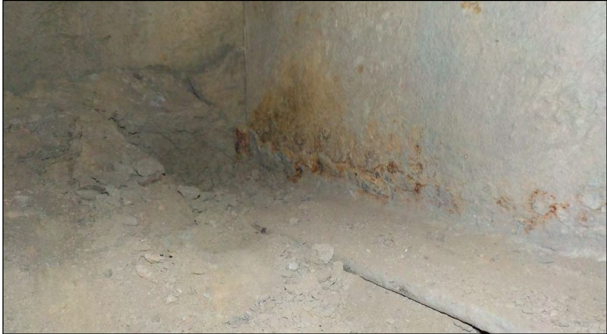
Photo 46: Span 1, Abutment 1, Stringer 5: the stringer web had heavy corrosion and up to 50 percent section loss over a 10 in. long by 1 in. high hole adjacent to the stringer end
