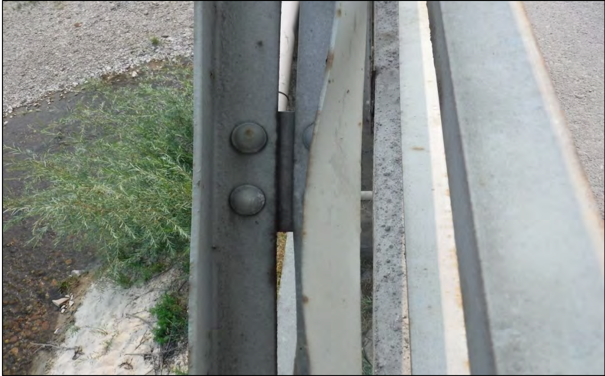
Photo 74: Span 2, North Truss, Diagonal L2'-U1': the interior flange was bent 1-3/8 in. over a 24 in. length due to impact damage
