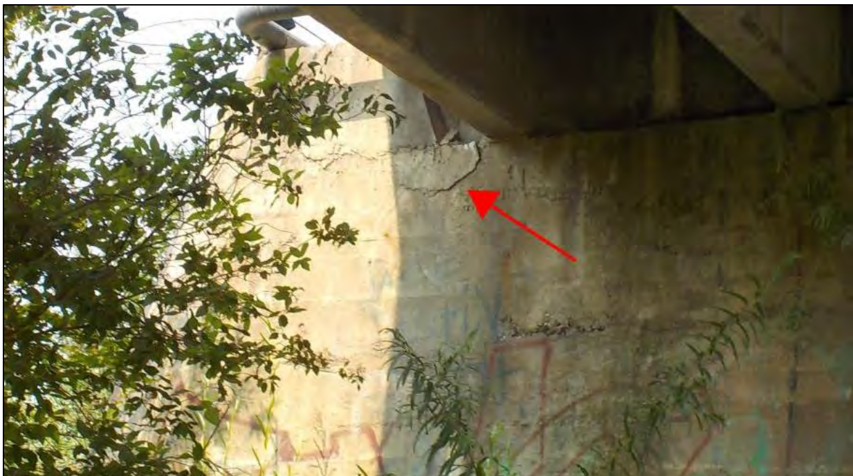
Photo 57: Bent 3 had a 12 in. wide by 10 in. high area of delamination on the top, southeast corner of the bent
