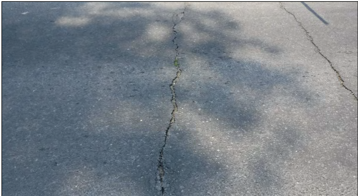
Photo 21: 1/2 in. wide transverse crack located 4 ft. from the East Transition
