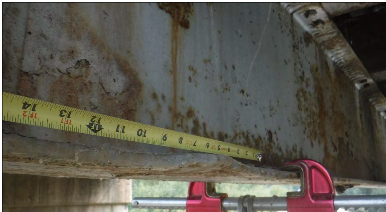
Photo 43: The bottom west flange of Floor Beam 1' on Span 1 had bent upwards 1/2 in. over a 6 in. length approximately 16 in. from the north end
