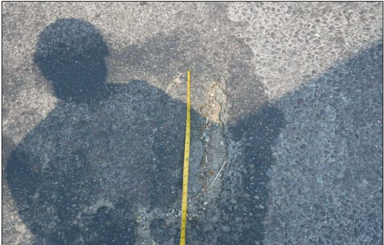
Photo 23: Typical minor wear on Span 1 bituminous overlay
