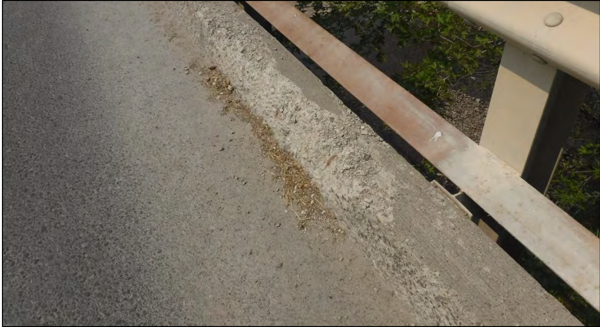
Photo 30: The North Curb on Span 4 had section loss up to 1-1/2 in. on the top and interior faces with no exposed reinforcing steel
