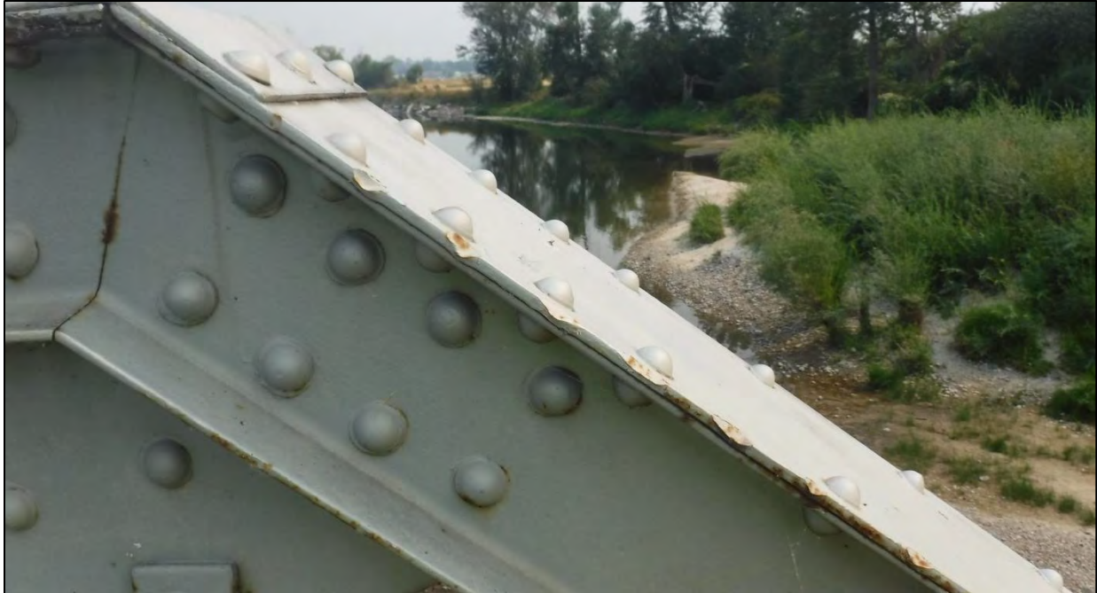
Photo 76: Span 2, North Truss, Diagonal L0'-U1': the diagonal had seven areas of impact damage up to 3/4 in. long and 1/4 in. of deflection spaced over a 15 in. length
