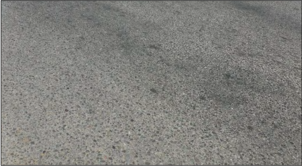
Photo 18: Minor wear to West Approach. Similar condition on East Approach
