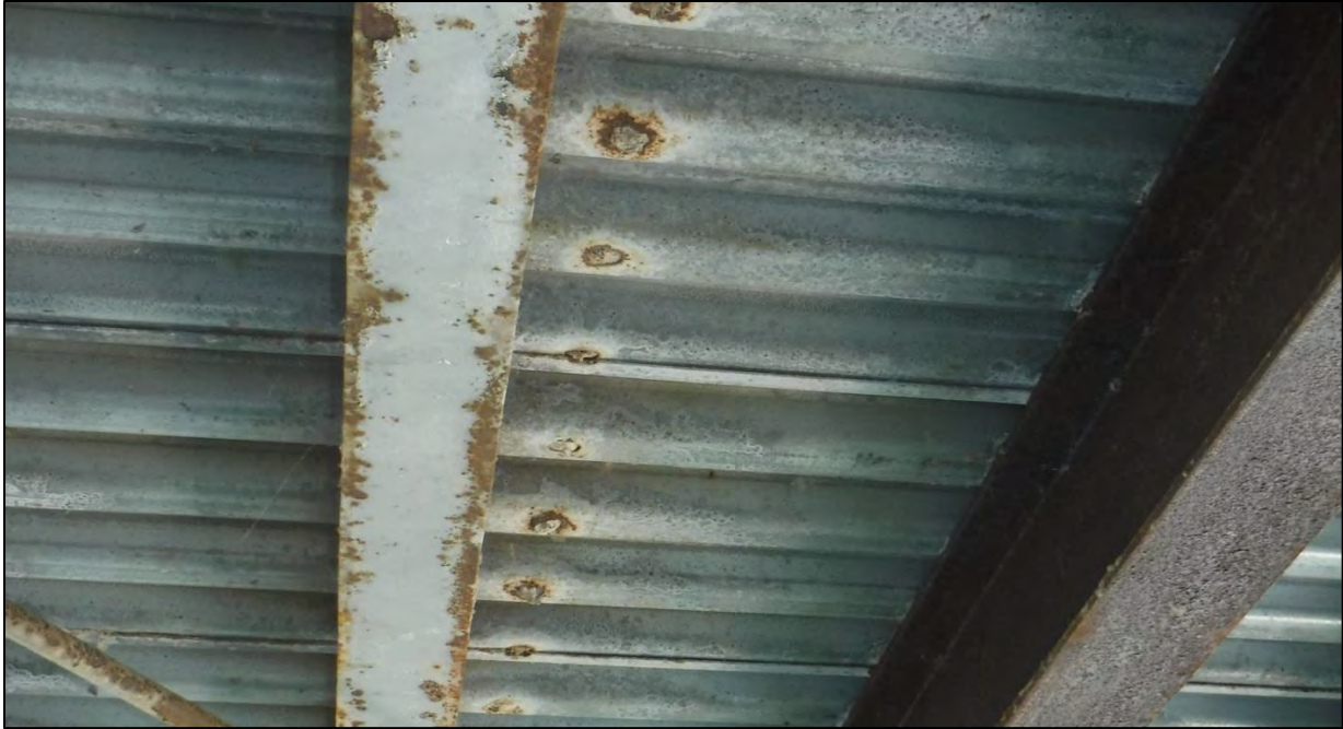
Photo 28: Typical underside of Span 1 deck; Note burn through holes in corrugated steel
