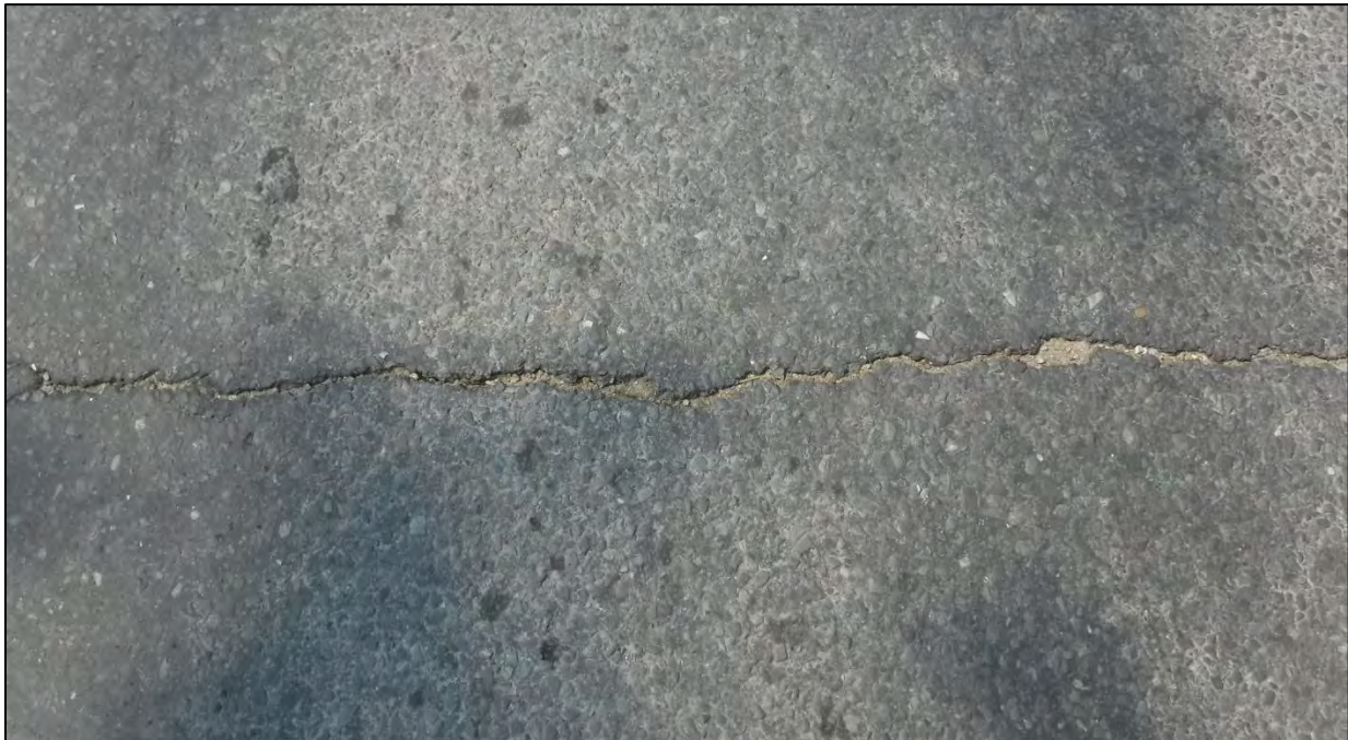
Photo 27: Transverse crack up to 1/2 in. wide over Abutment 5
