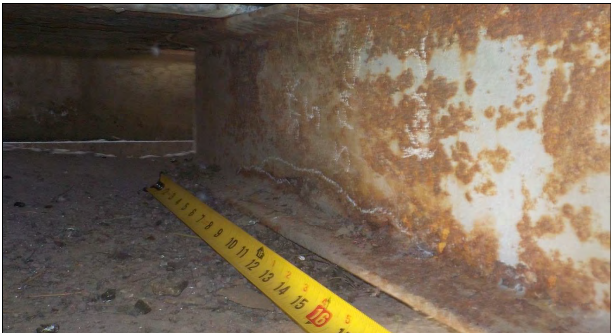
Photo 49: Span 2, Bent 2, Stringer 5: the south face had a 16 in. long by 2 in. tall area of pack rust up to 1/4 in. thick on the bottom of the web located 12 in. from the end of the stringer
