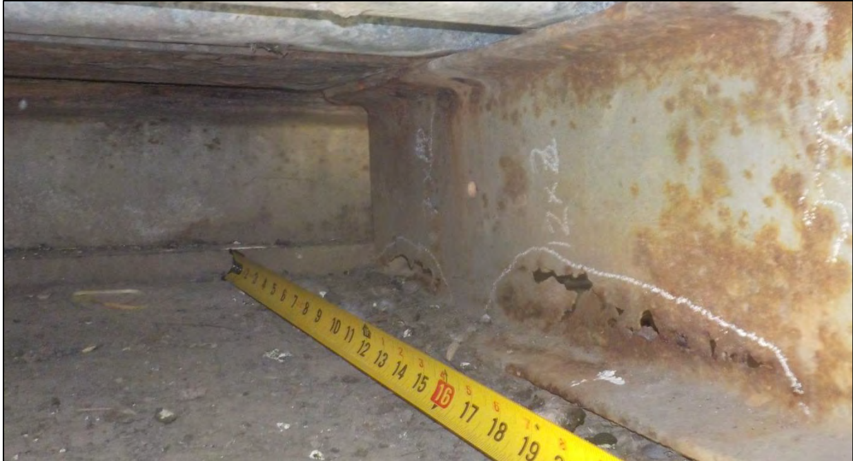
Photo 48: Span 2, Bent 2, Stringer 2: the stringer web had heavy corrosion and section loss with two holes; 7 in. long by 1 in. high and 6 in. long by 2 in. high centered 16 in. from the stringer end
