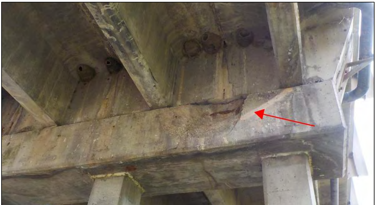
Photo 59: Bent 4 had a 3 ft. wide by 2 ft. high spall with exposed reinforcing steel on the west face of the bent cap. The exposed reinforcing steel had moderate corrosion with negligible section loss
