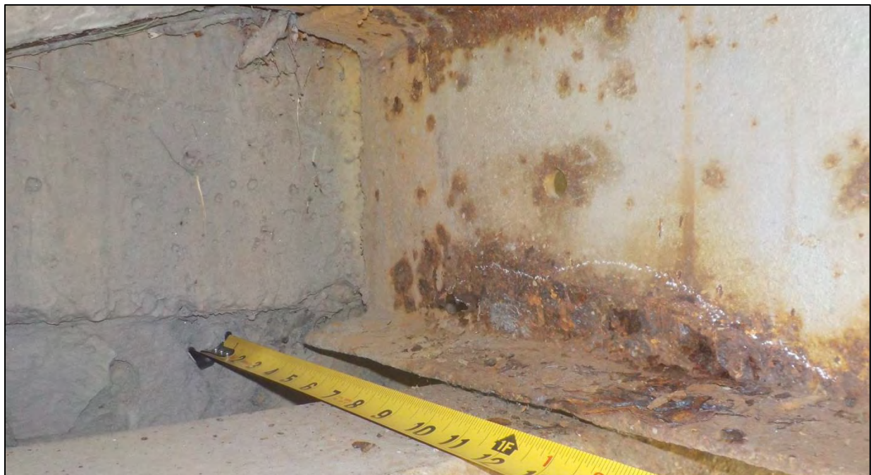
Photo 53: Span 2, Bent 3, Stringer 7: the stringer web had heavy corrosion with up to 50 percent section loss over a 6 in. long by 2 in. high adjacent to the stringer end that had a 1/2 in. diameter hole 6 in. from the stringer end at the web to lower flange interface
