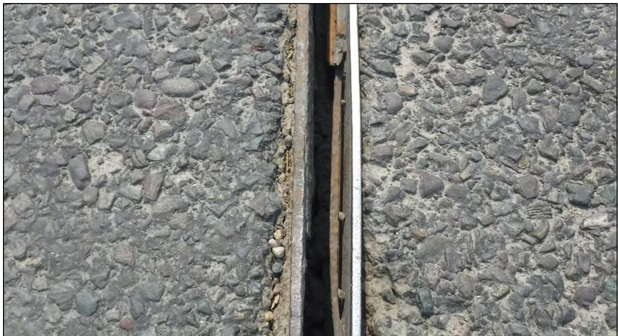
Photo 41: Joint 3 over Bent 3 with seal deterioration which was typical over 90 percent of the length
