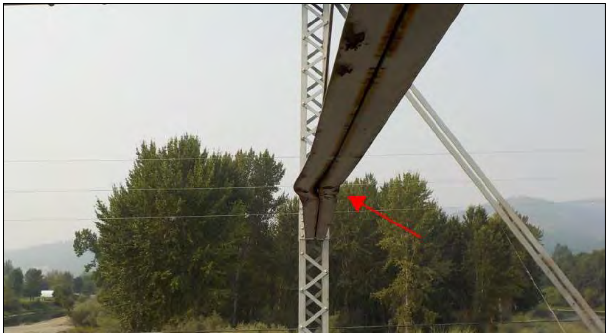
Photo 77: Panel Point 3': the lower, horizontal bracing member was bent 2 in. to the east, and bent upward and downward 1 in. due to impact damage
