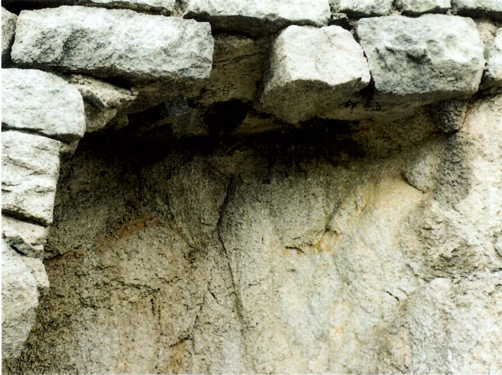
PHOTO 5: Harding Way Retaining Wall (24SB1163), close up of foundation of retaining wall
