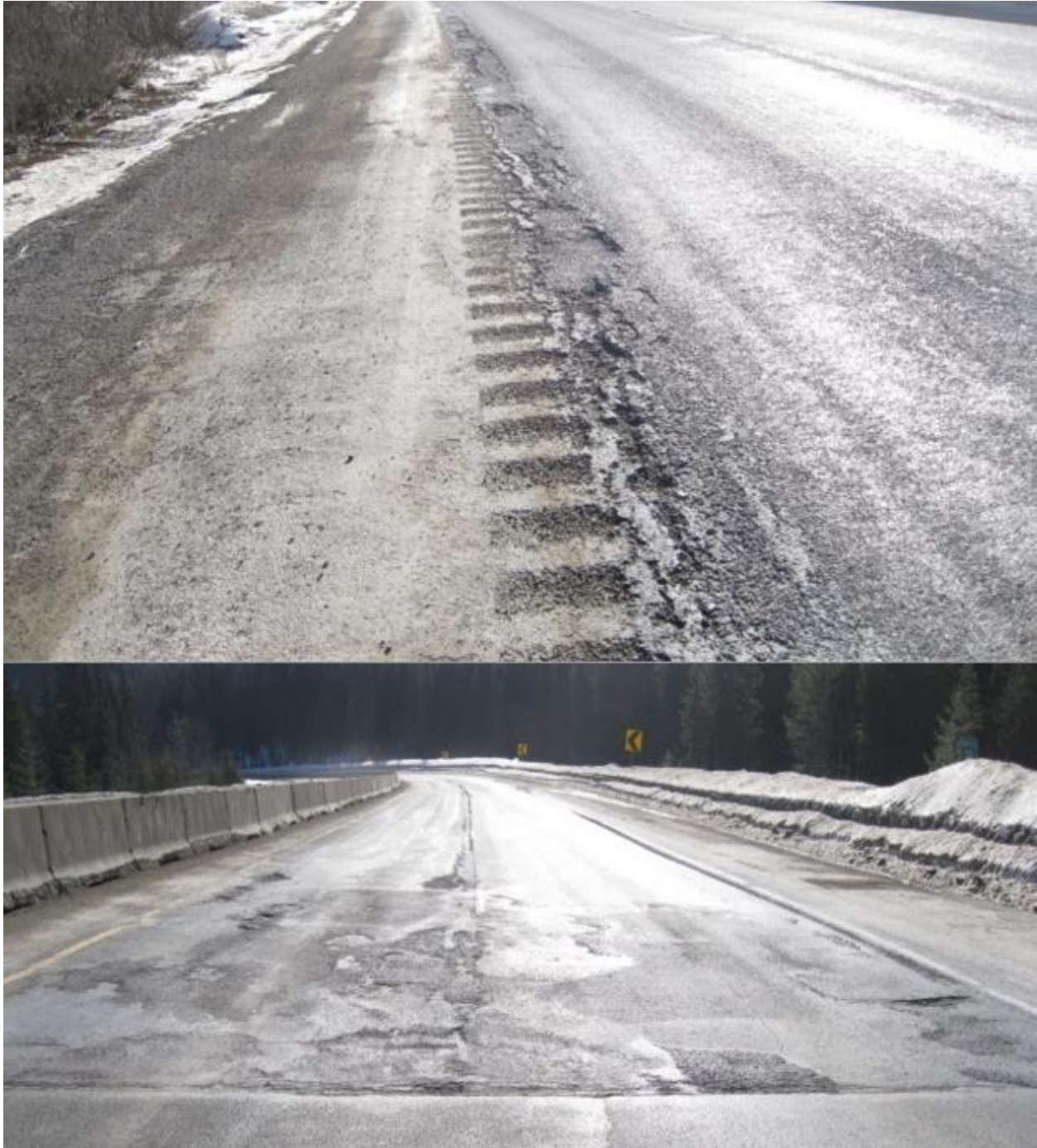
Figure 2 – Pavement distress visible at the surface, March 2020
