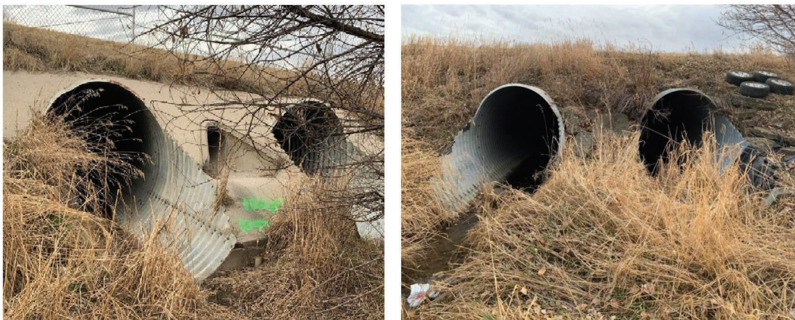
Figure 3-3. Box Elder Creek, Dual 84-in. CSP Entrance and Exit
