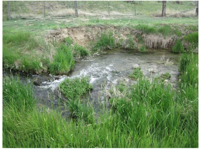
Photo 2 Desc: Grade control and eroding bank downstream of Hwy 41.
