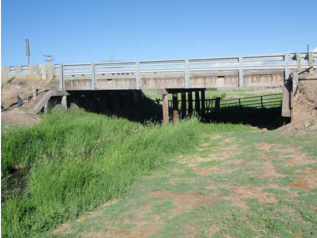
Photo 49 Bearing: W Location: RM 9.02 Desc: Potential location for wildlife underpass, could be incorporated into Stone Creek Bridge design.
