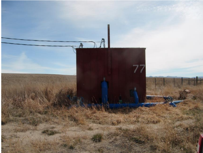
MP 10.8, east side road – irrigation pump station
