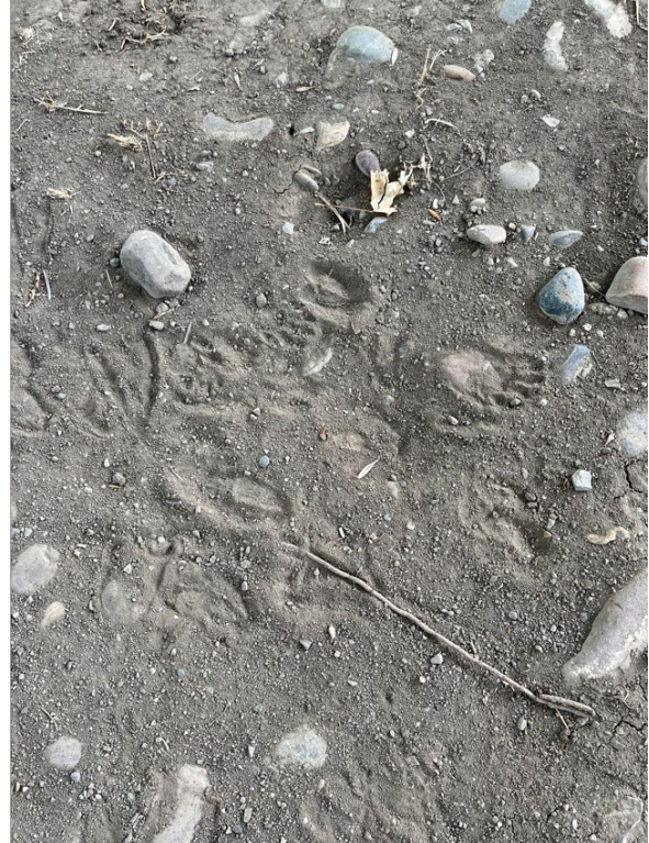
Photo 6: Animal tracks in dirt underneath the east bridge abutment.
