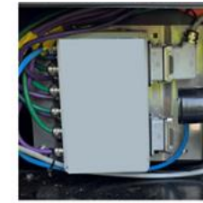
a. Junction Box
