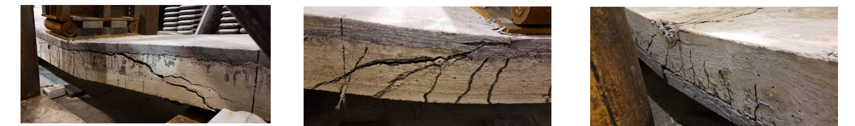
O-PR1 Shear crack widening/spreading
