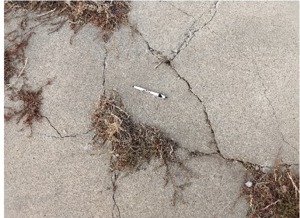
A-1, Shattered Slab
