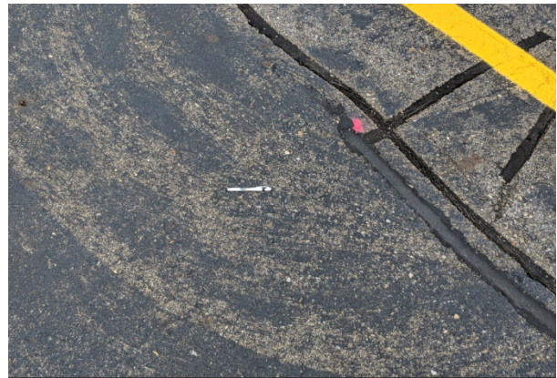
A-1, Dense Grade - Raveling
