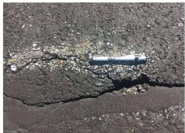
R-3, Crack with Mechanical Raveling
