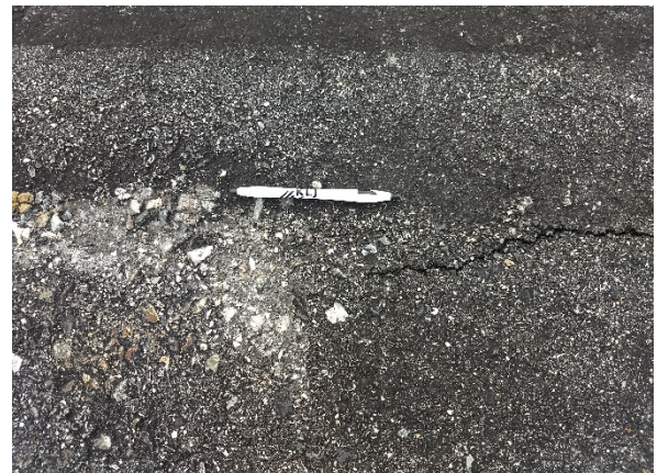
T-2, Crack with Mechanical Raveling
