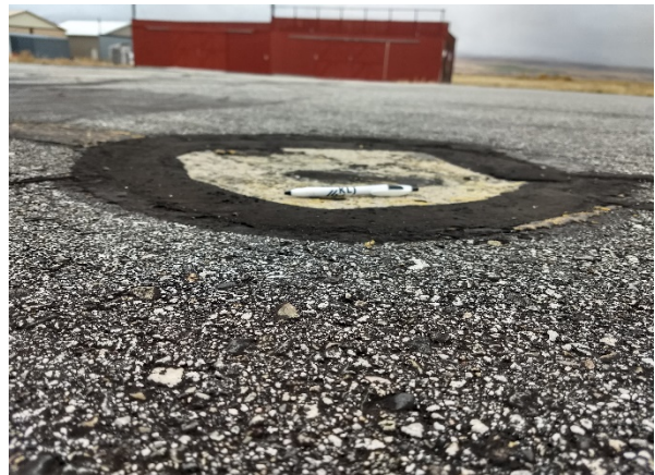
A-3, Patch Depression and Crack
