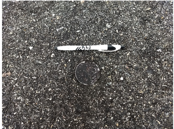
T-1B, Surface with Duct Marker
