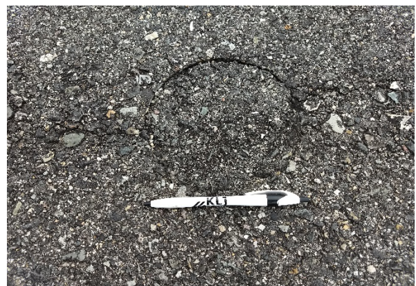
A-4, Surface, Patch and Crack
