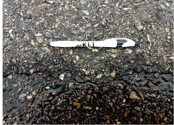
A-3, Surface with Crack
