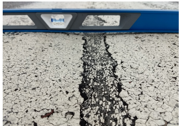
R-3, Crack and Depression
