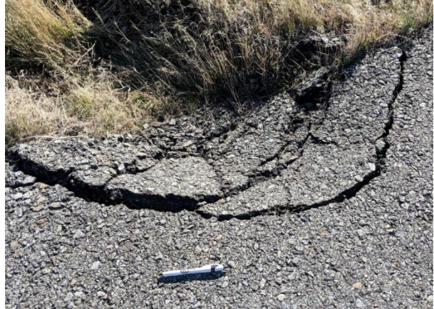
T-1, Major Crack Depression
