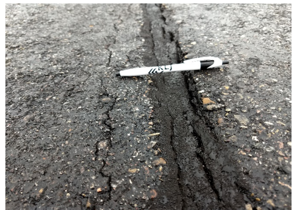
R-11, Parallel Cracks
