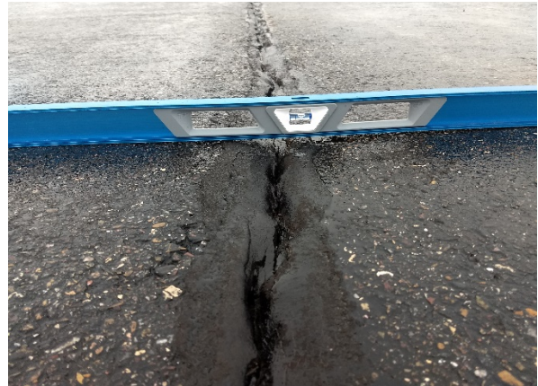
A-11, Crack with Failed Sealant
