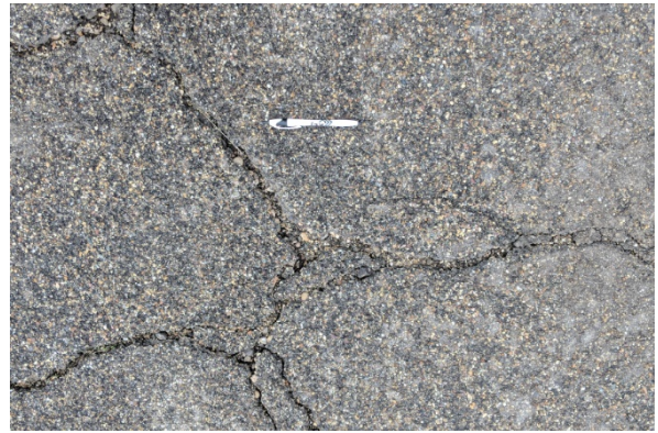
T-1B, Block Crack
