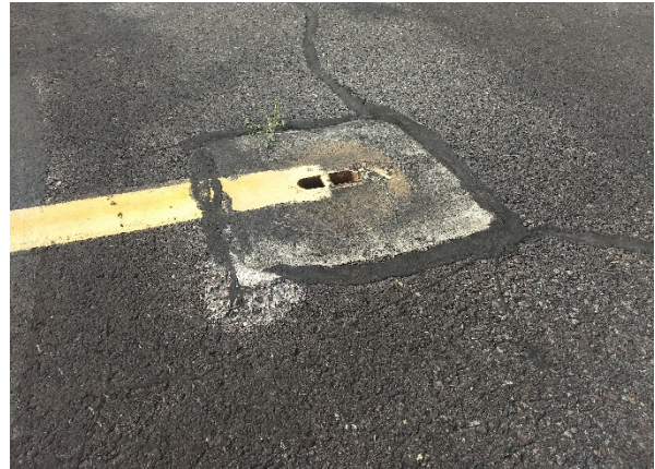
A-11, Tie Down with Sealed Crack
