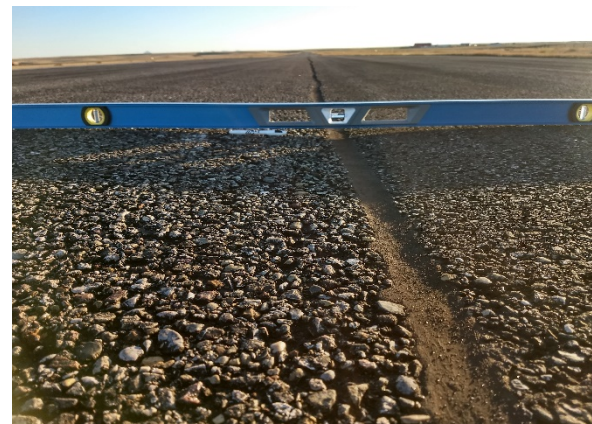
R-21, Sealed Crack and Depression
