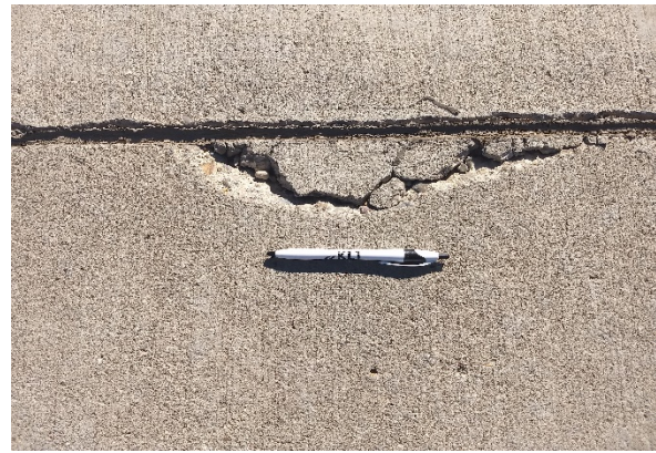
A-22, Joint Spall
