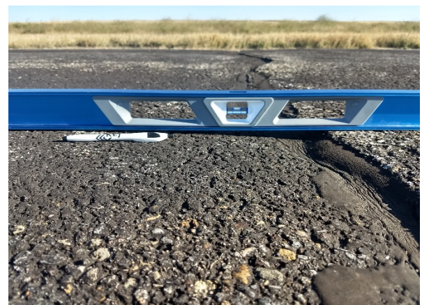
T-21, Sealed Crack and Depression
