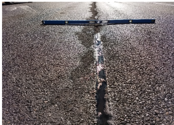
R-1, Crack and Depression
