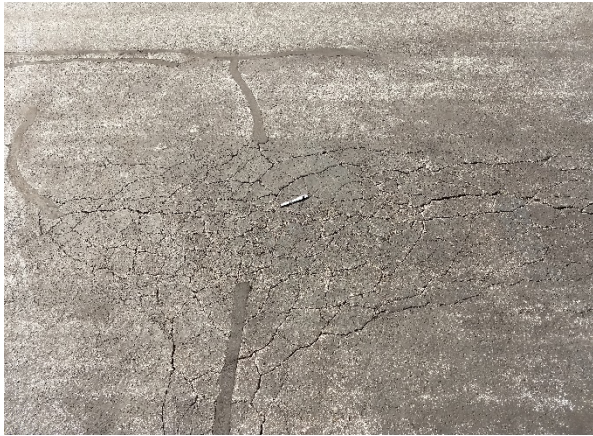
A-2, Alligator Cracking
