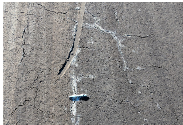
T-1, Block Crack
