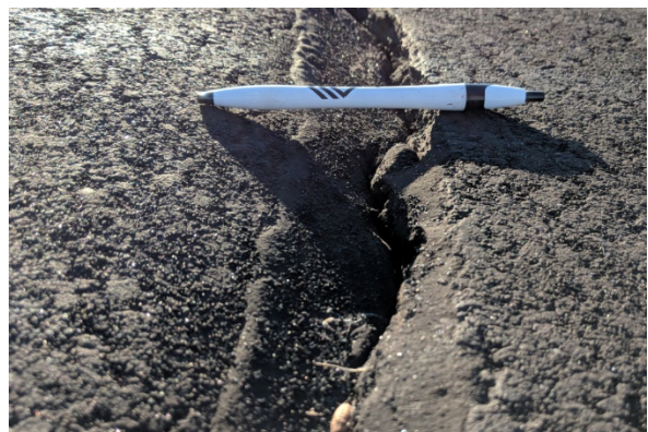
R-11, Crack with Depression
