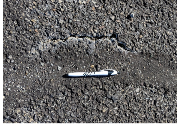
T-1, Crack Sealed
