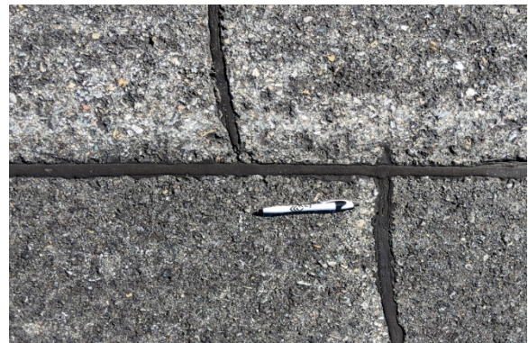
R-11, Surface Cracks
