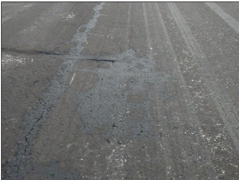
RW06-01-68: Alligator Cracking
