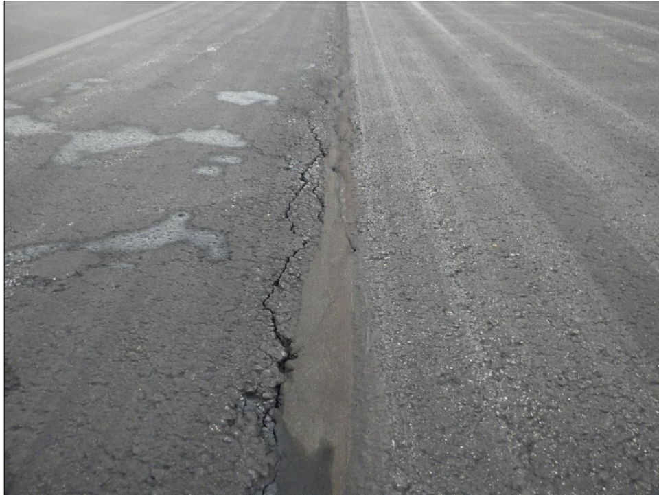
RW06-01-20: L&T Cracking
