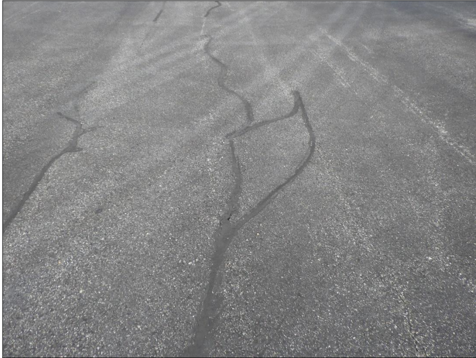
AP01-01: L&T Cracking
