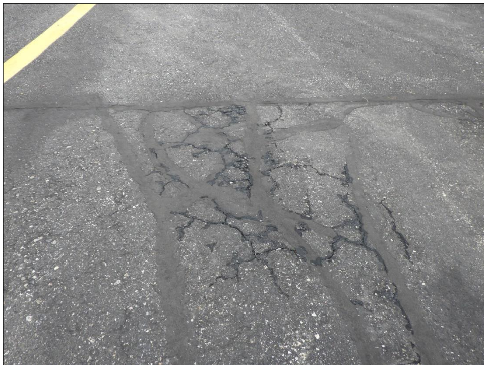
TW02-07: Alligator Cracking
