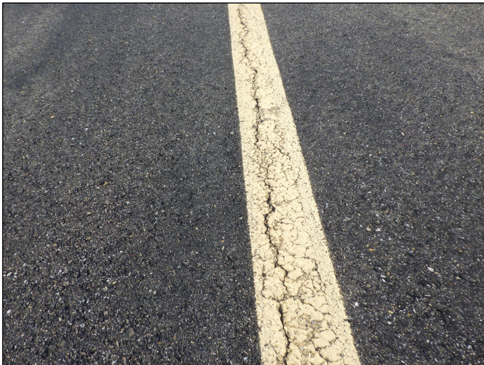
TW01-07: L&T Cracking
