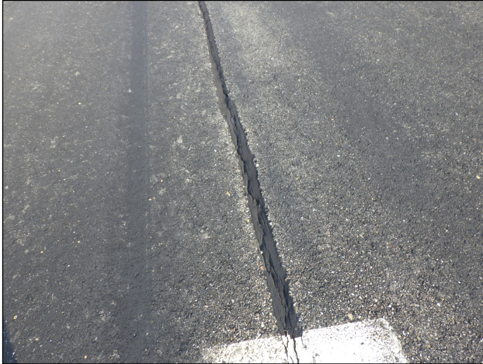
RW10-01-46: L&T Cracking
