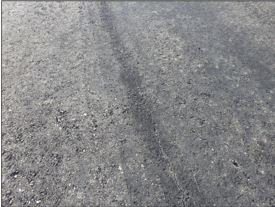
AP01-06: L&T Cracking
