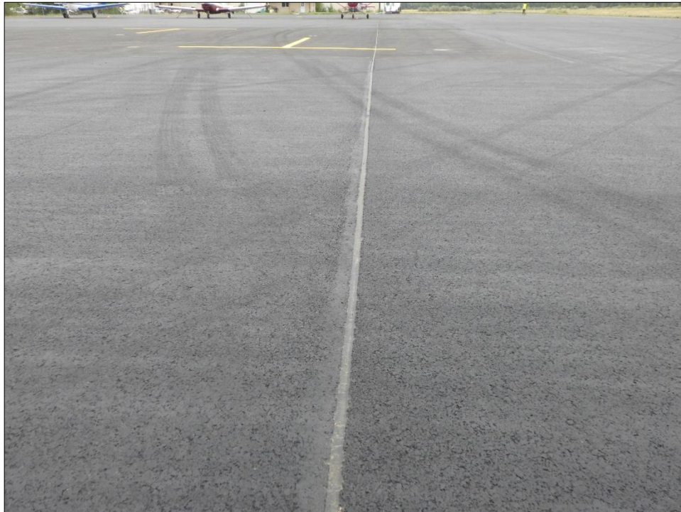
AP11-07: L&T Cracking
