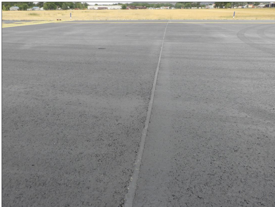
TW11-17: L&T Cracking
