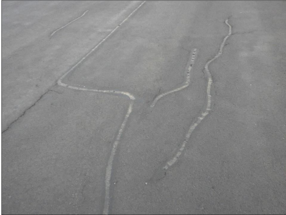
AP01-02: L&T Cracking
