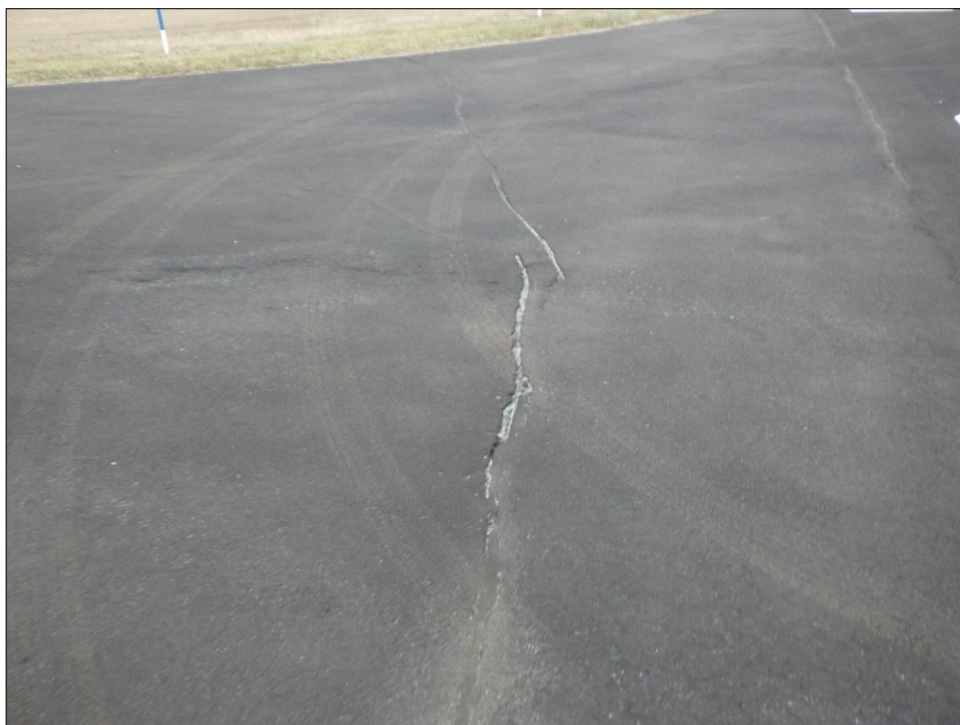
TW02-01: L&T Cracking
