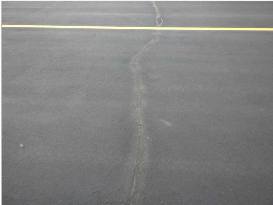
TW01-02: L&T Cracking
