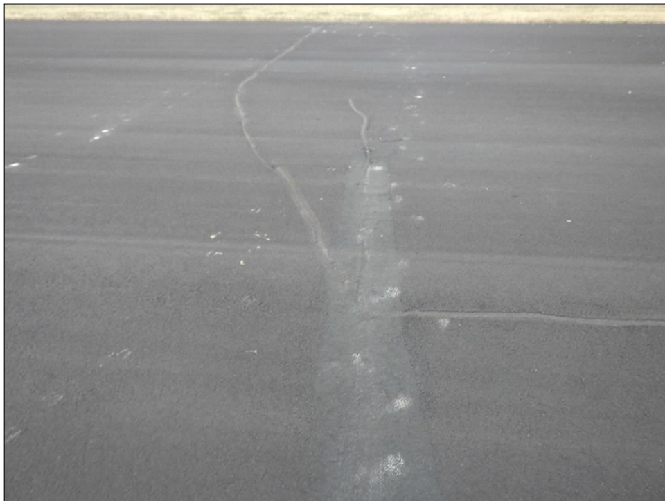
RW08-02-02: L&T Cracking
