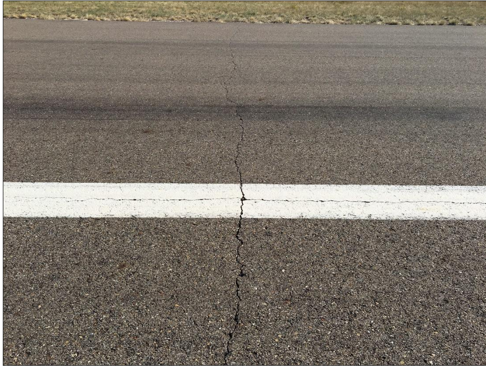
RW11-50: L&T Cracking
