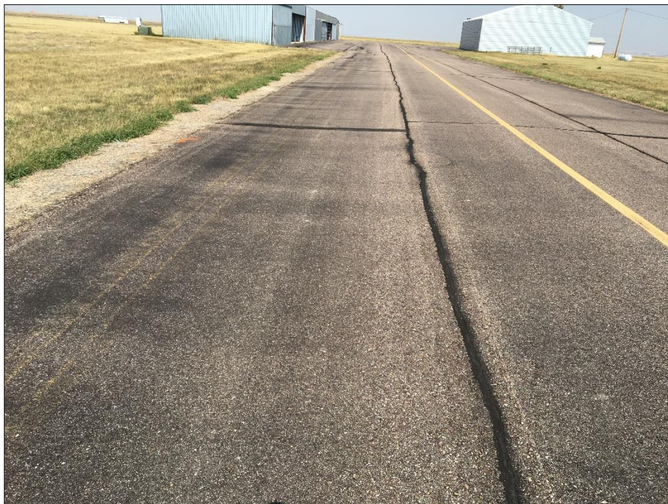
TW05-10: L&T Cracking
