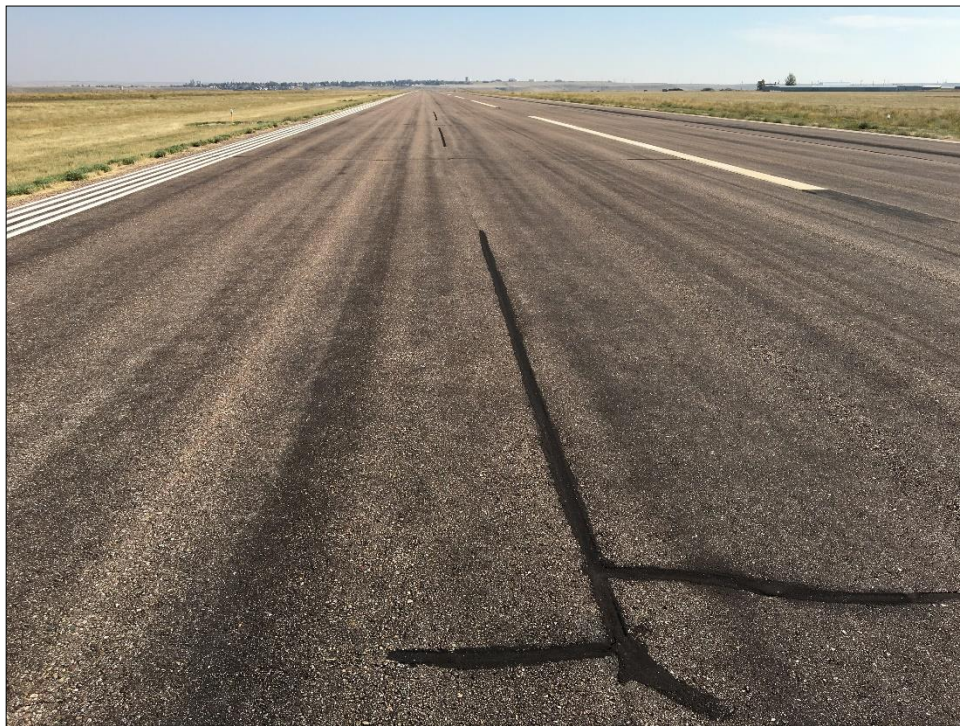
RW21-41: L&T Cracking
