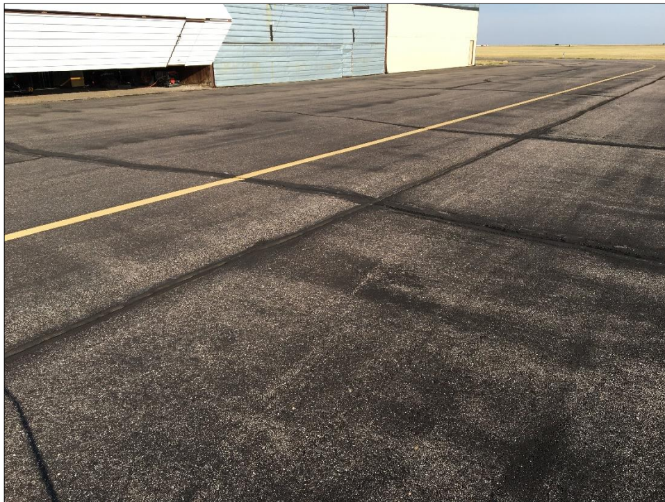
TW05-02: Overview, L&T Cracking
