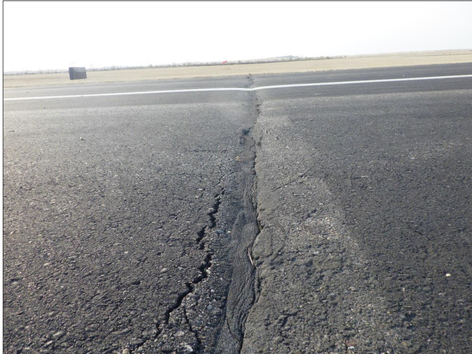
RW02-03-18: L&T Cracking
