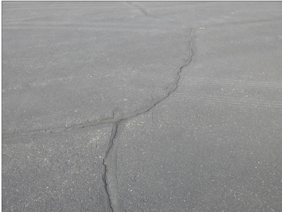
AP01-21: L&T Cracking
