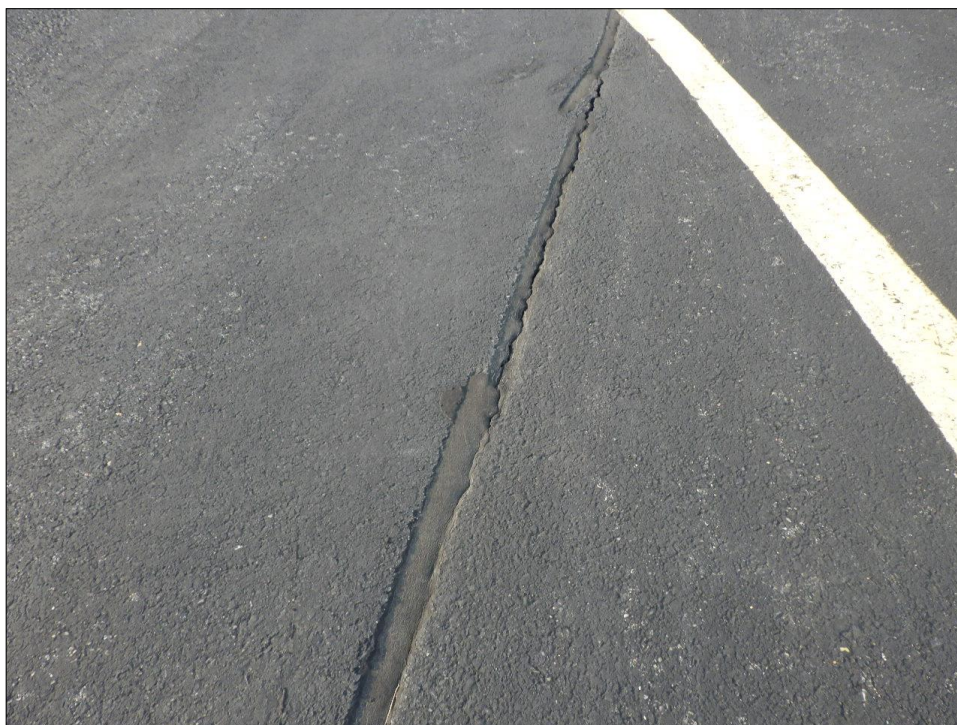
TW12-02: L&T Cracking
