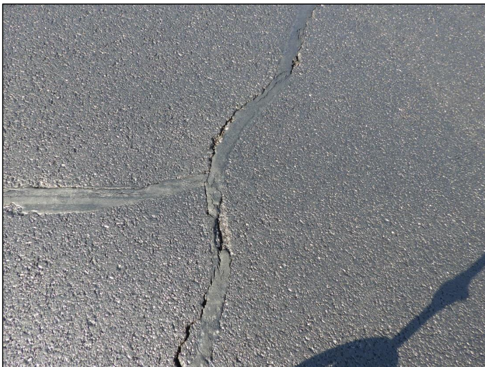
AP03-07: L&T Cracking
