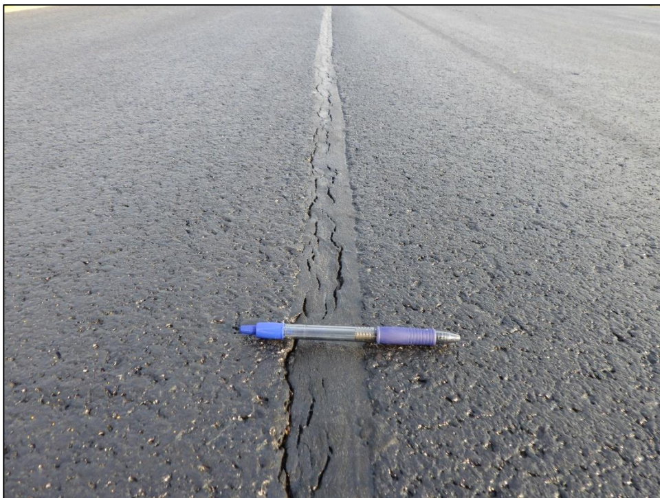
TW05-04: L&T Cracking
