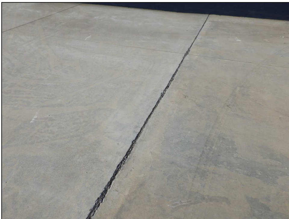
AP06-02: Joint Spalling
