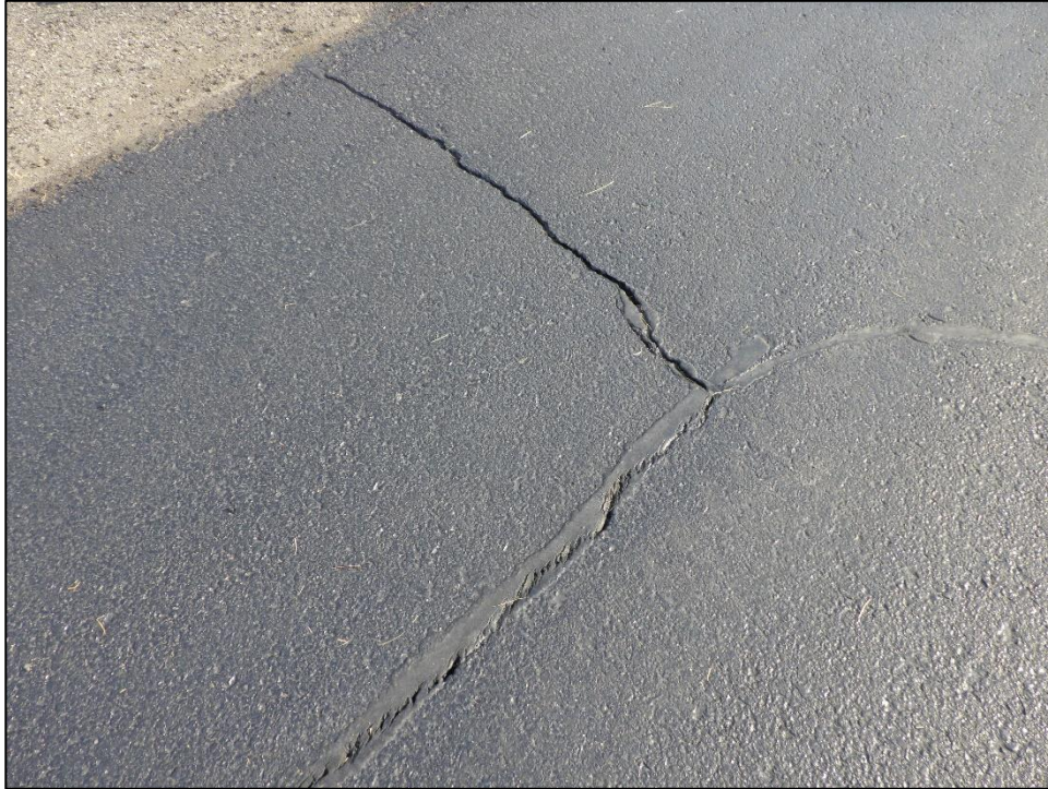
TW03-02: L&T Cracking
