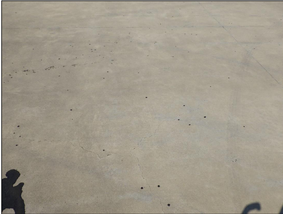
AP04-01: Shattered Slab/Intersecting Cracks
