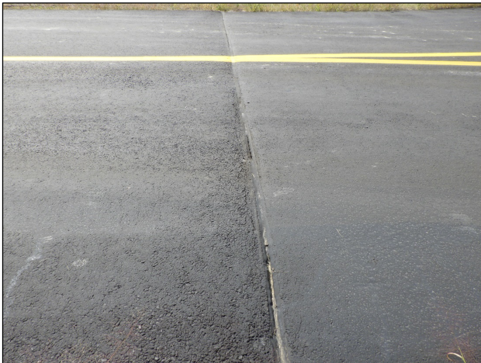
TW02-04: L&T Cracking
