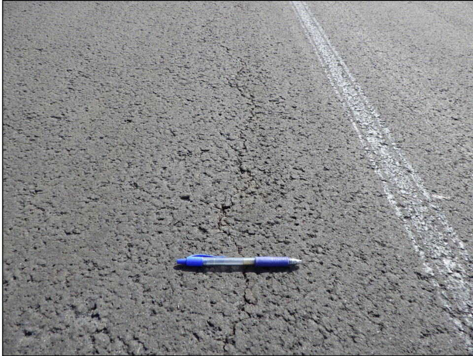
RW13-01-21: L&T Cracking
