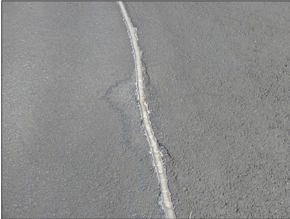
AP01-05: L&T Cracking
