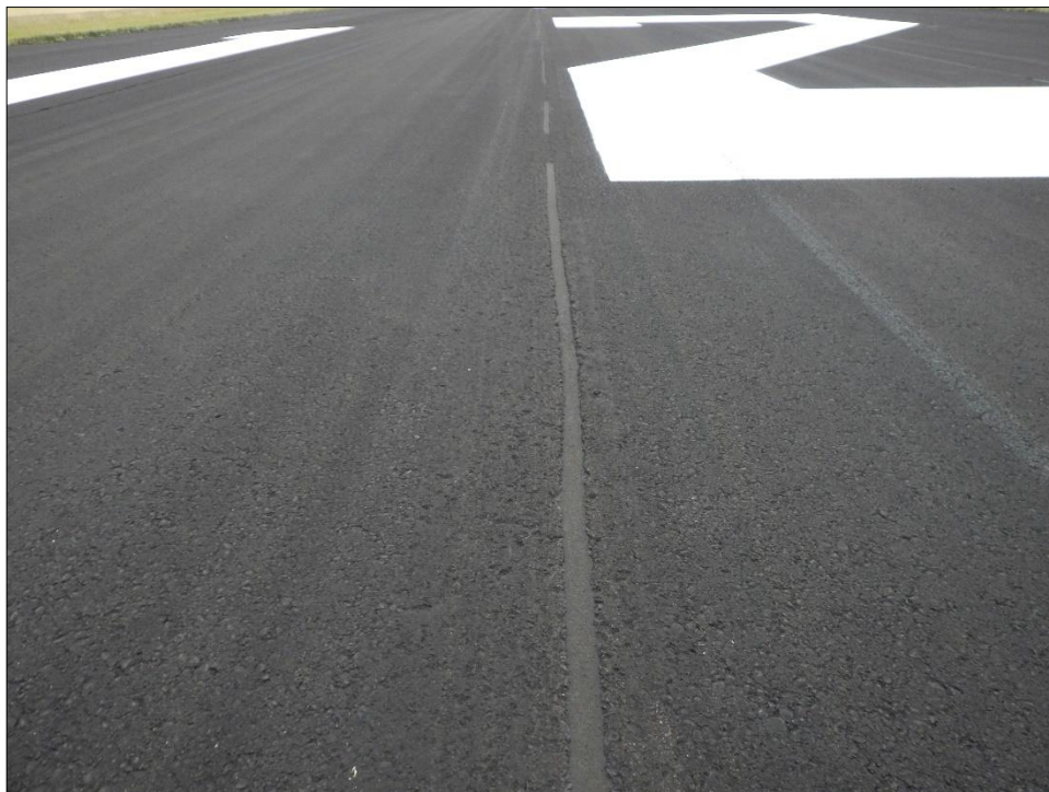
RW12-11-04: L&T Cracking
