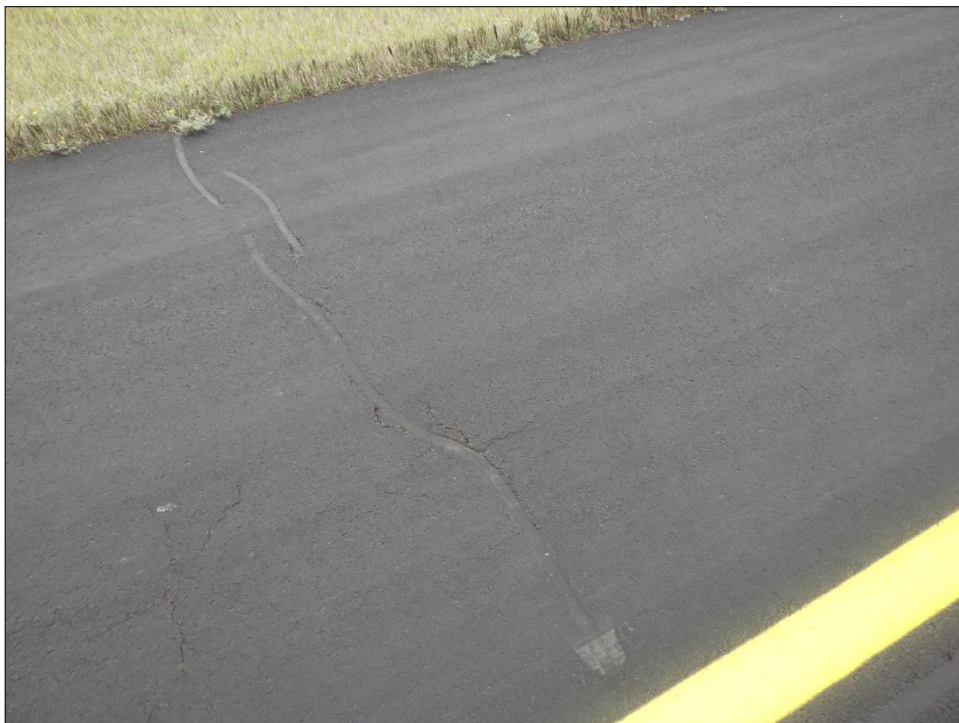
TW11-24: L&T Cracking
