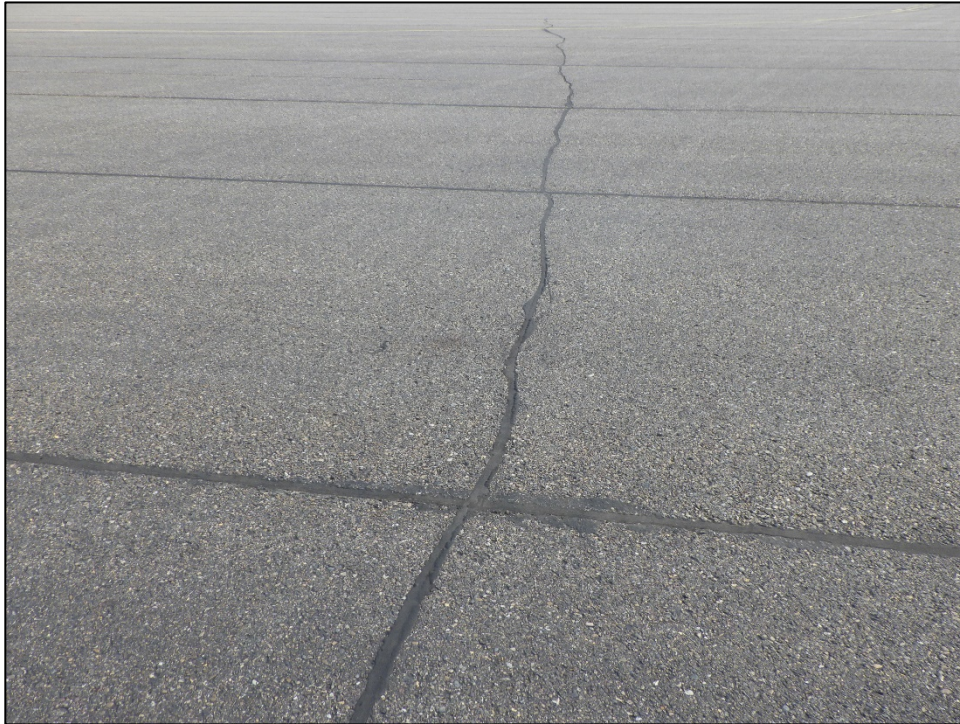
AP03A-03: L&T Cracking
