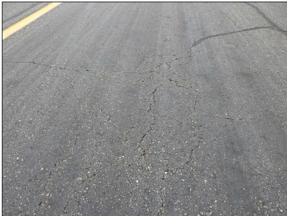
TW05-01: Alligator Cracking
