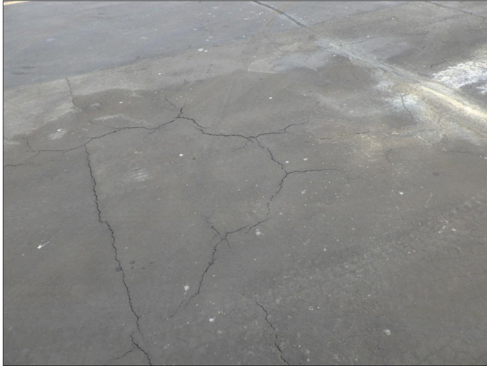
AP01-06: L&T Cracking
