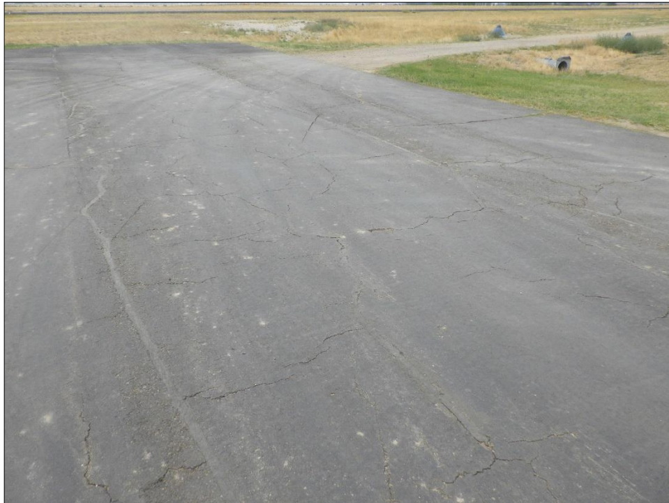
AP01-01: Block Cracking
