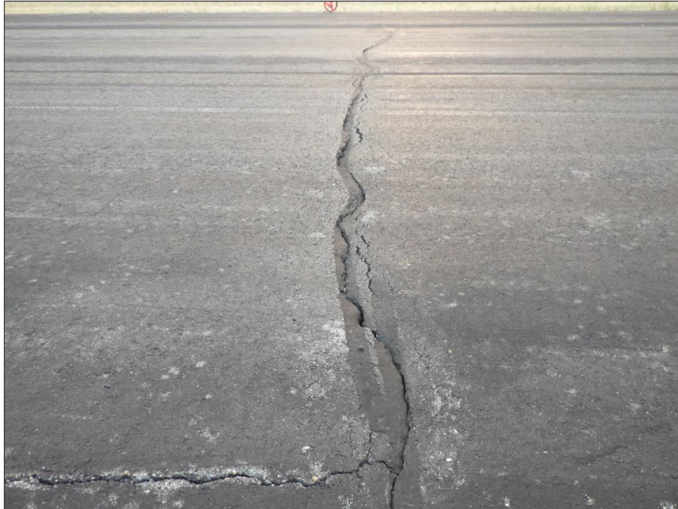
RW17-01-11: L&T Cracking
