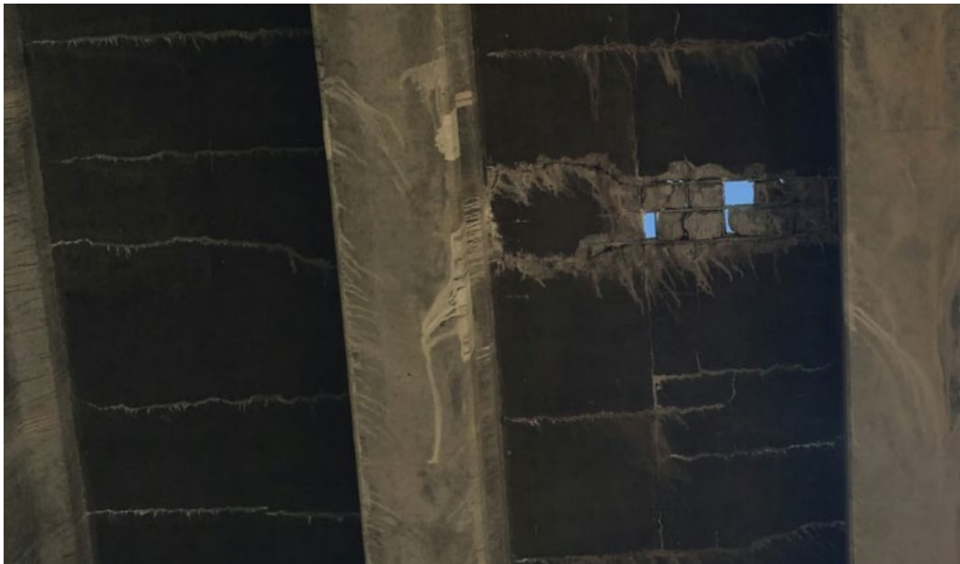
Figure 5. Same hole as Fig. 4 as seen from Underneath. Note the heavy staining on the soffit and girders from leakage in the cracks around the hole and in nearby transverse cracks. Note, little or no staining in cracks in adjacent girder bay. Note jump cracks with beginning staining at another location not far from the hole.
