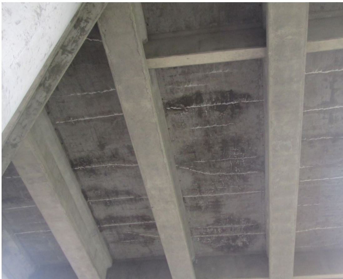
Figure 3. Typical Transverse Cracks Seen From Underneath
