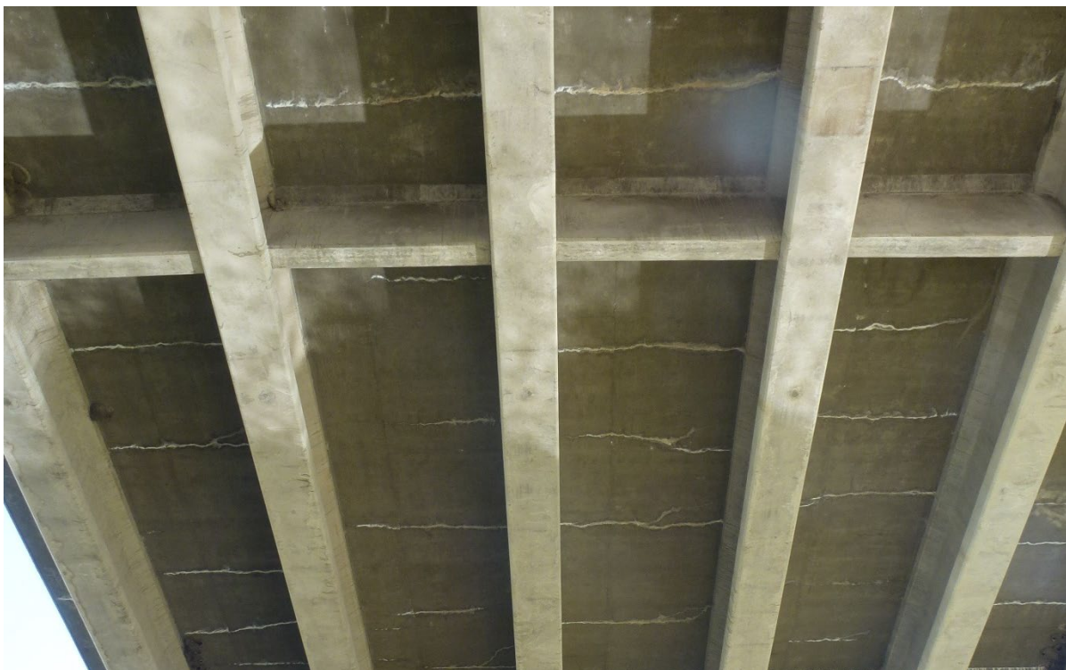
Figure 8. Example of Condition State 2. Note possible beginning jump cracks
