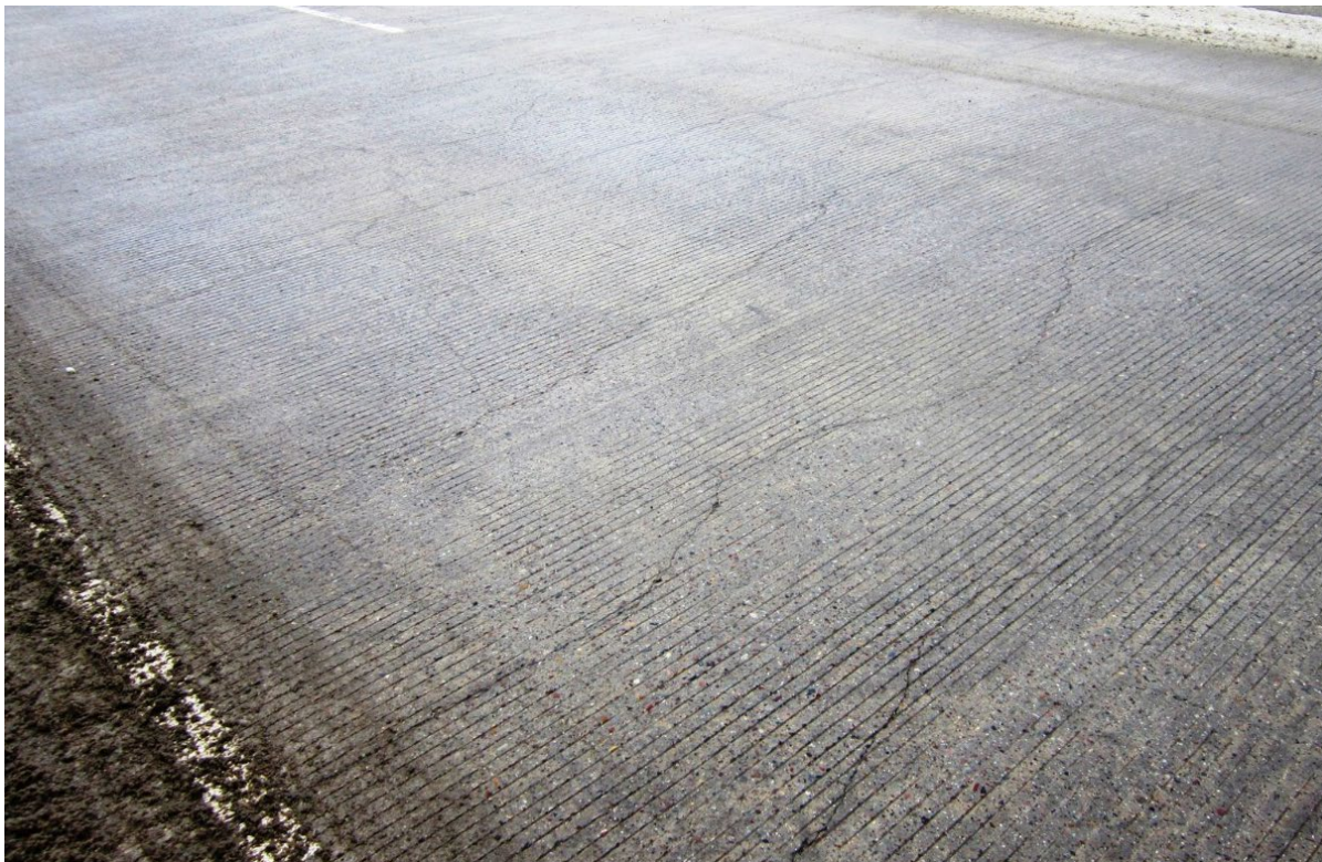
Figure 2. Transverse Cracks in Bridge Deck
