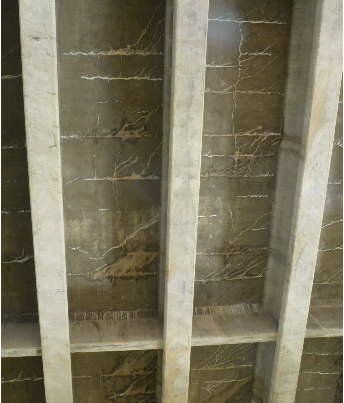
Figure 11. Example of Condition State 4. Note the tight spacing, multiple jump cracks (some creating the concrete "islands"), very heavy gray staining and efflorescence.
