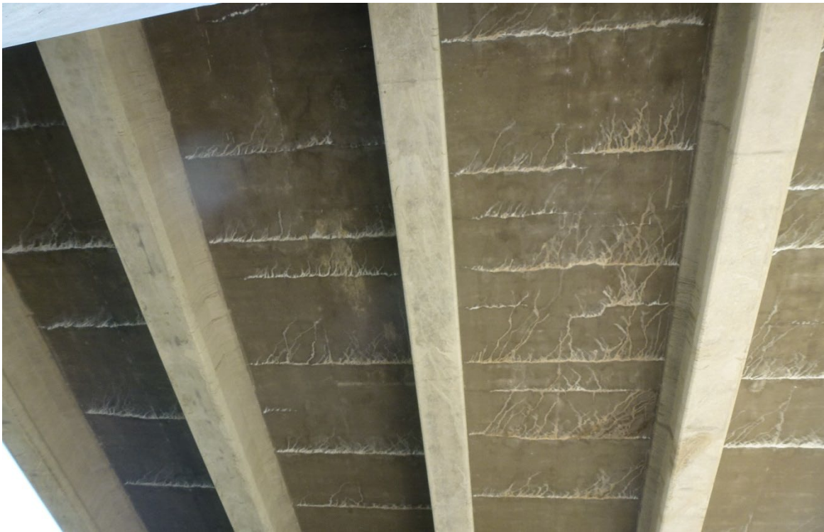
Figure 9. Example of Condition State 3. Note the tight spacing (12" to 18") of some of the transverse cracks, along with evidence of heavy leakage and some gray efflorescence. Also, small jump cracks evident.
