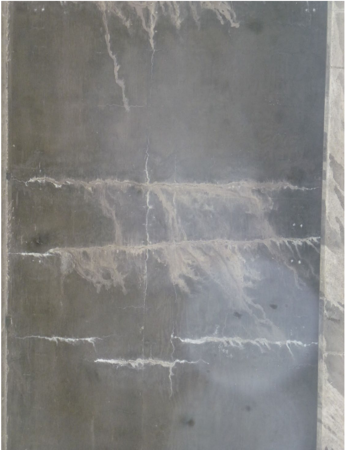
Figure 6. Example of Heavy staining from water leakage. Note the contrast between the gray efflorescence in the upper 2 transverse cracks (evidence of concrete movement around crack and heavy water leakage) and the white efflorescence in the bottom transverse cracks. Note the longitudinal jump crack with light white efflorescence.
