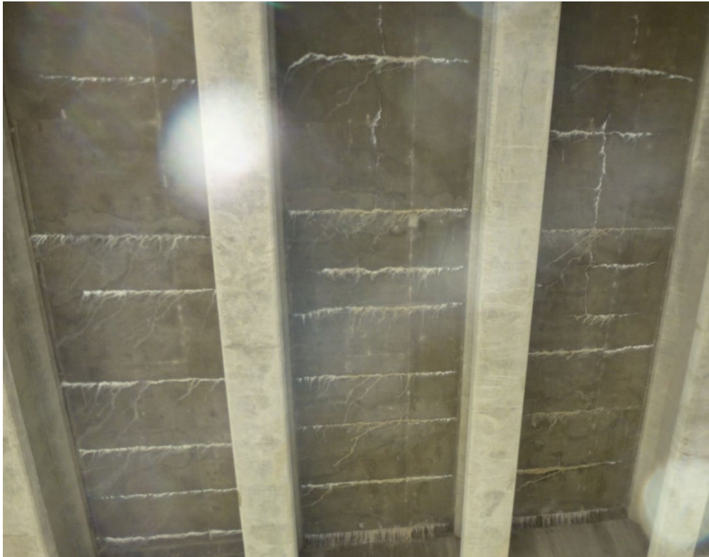
Figure 10. Example of Condition State 3. Tight spacing, jump cracks, some light staining from leakage, and some gray efflorescence.
