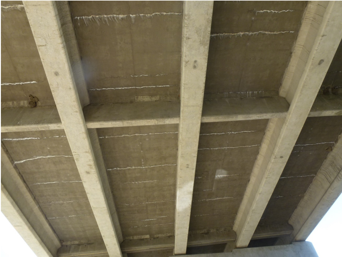
Figure 7. When to not use the transverse pattern cracking defect. Use the deck cracking defect only. Transverse cracking is present but sporadic. Note the wide crack spacing, the lack of staining, and no longitudinal jump cracks. All efflorescence is white.
