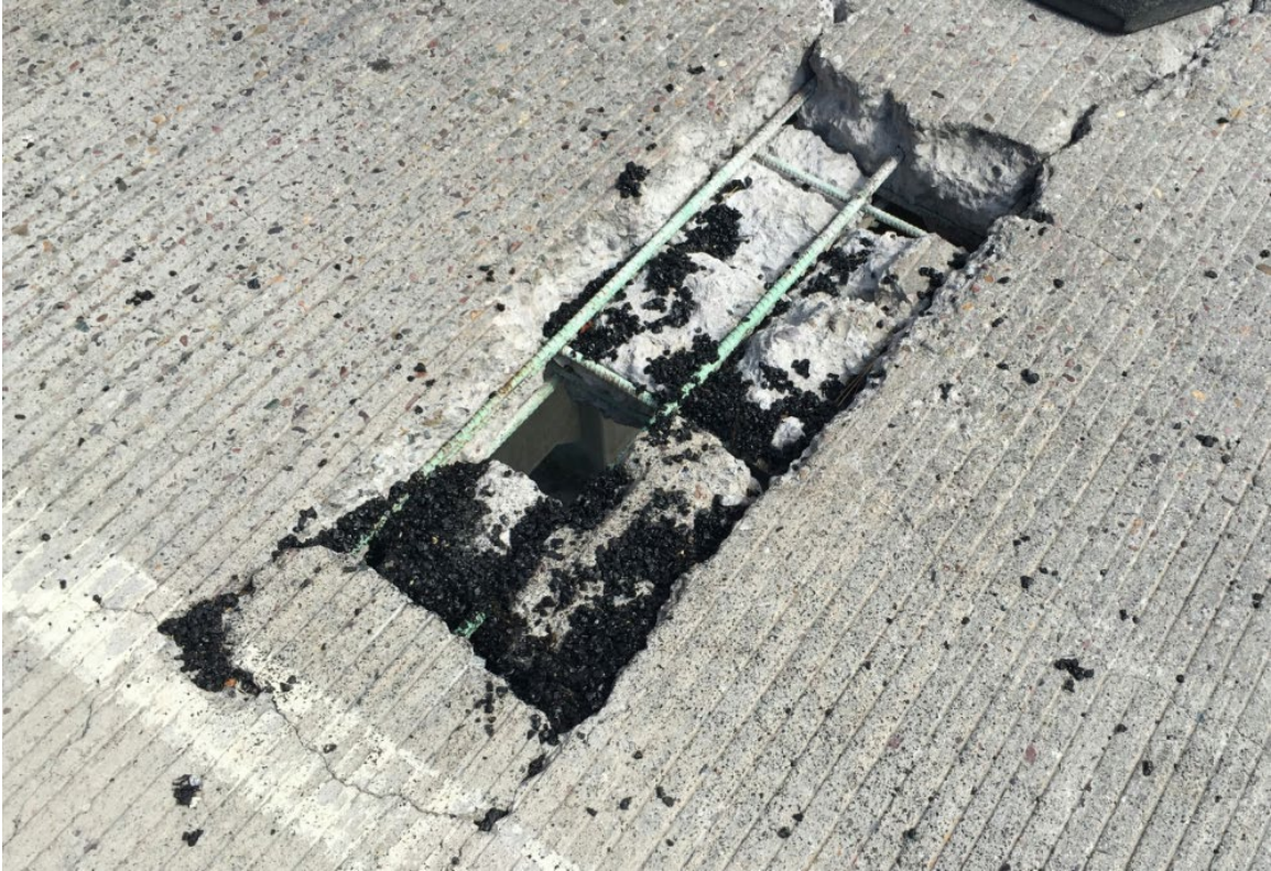
Figure 4. Holes in Bridge Deck. Note the longitudinal jump cracks that create the rectangular “island” of concrete. The “island” continued to crack until full depth chunk or “island” fell out, creating the hole.
